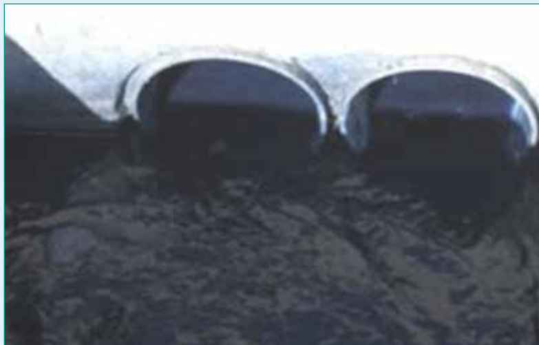
Fig. 2: The effluent from the plant shows extreme level of indigo pigment in the wastewater.
