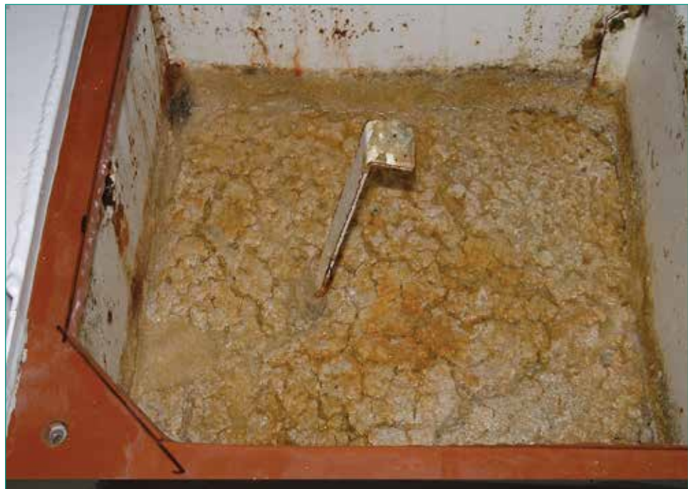
Fig. 1: "Before" treatment on 11/19/03 the grease trap was impacted with a thick grease cap.
