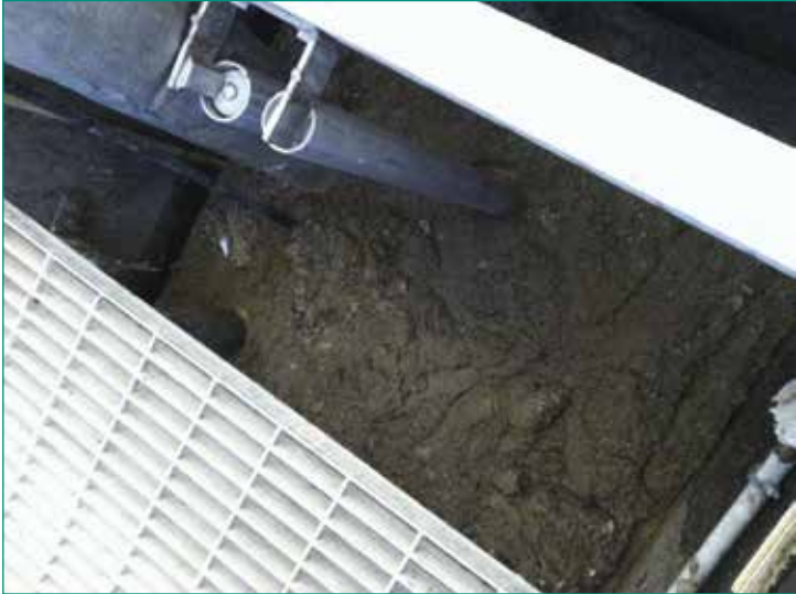
Fig. 1: With the grate open, a 2 - 3 foot grease layer is evident prior to treatment.
