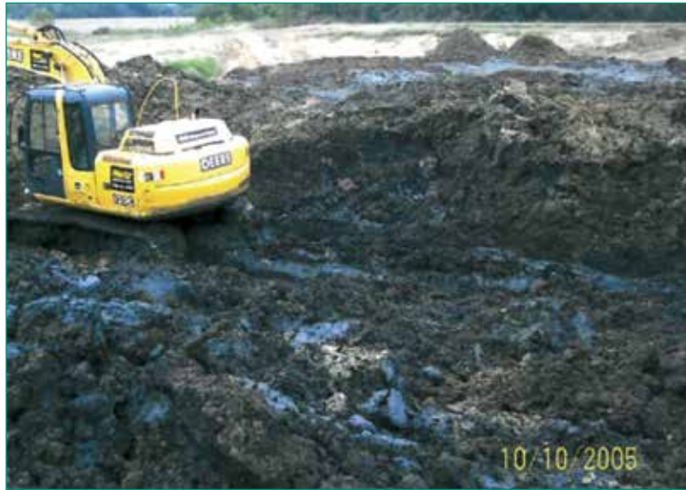
Fig 3: Excavation to ready the site for land farming shows the extent of contamination.
