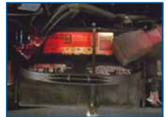
Battery with Protective Spray
