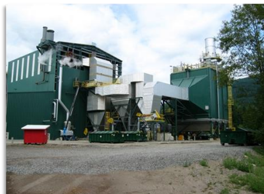
Wellons Steam Boiler
