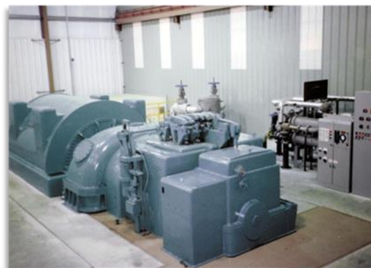
GE 10 MW Turbine Generator
