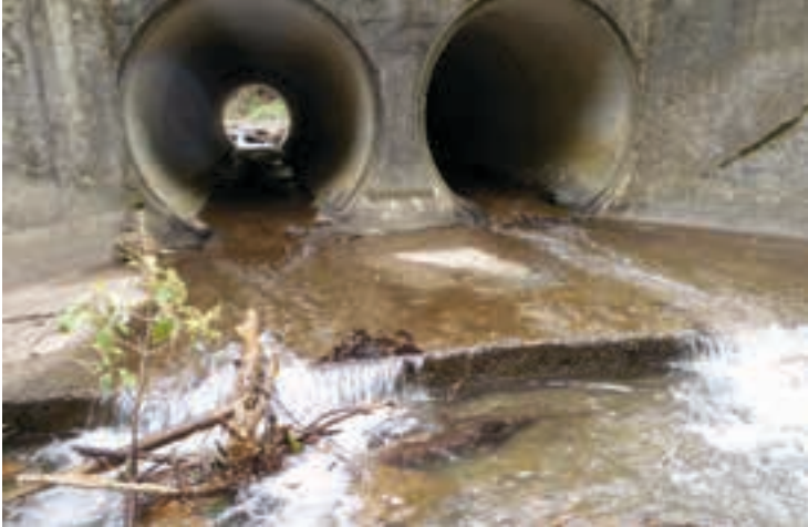
Poorly designed culverts are obstacles for migratory freshwater fish, preventing them from occupying habitats upstream
