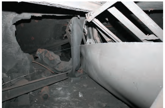
Photo 6. 1 North Longwall belt structure at a blown-out overcast. The belt structure has been completely overturned.
