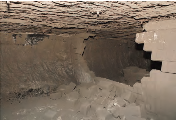
Photo 9. Stopping blown out toward the north as a result of the initial path of forces, at 73 crosscut, northeast of 78 switch.
