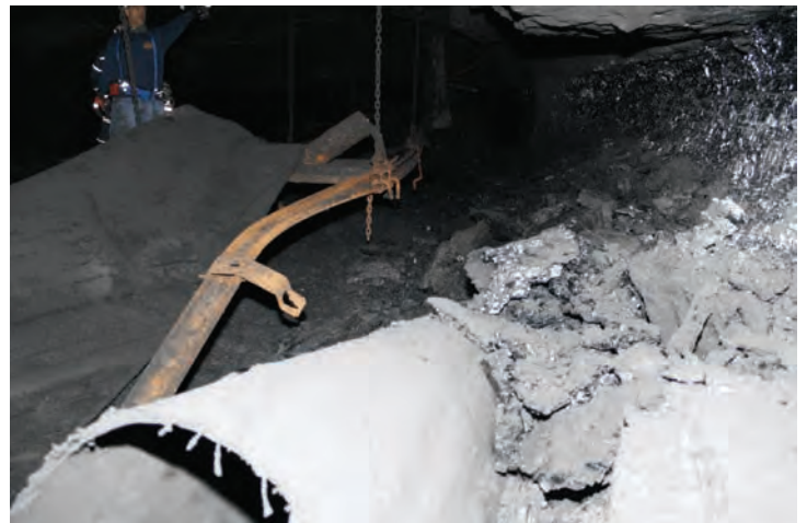
Photo 4. Bent and twisted steel belt structure at #4 crosscut of Tailgate 22 Section shows evidence from the forces of the explosion.
