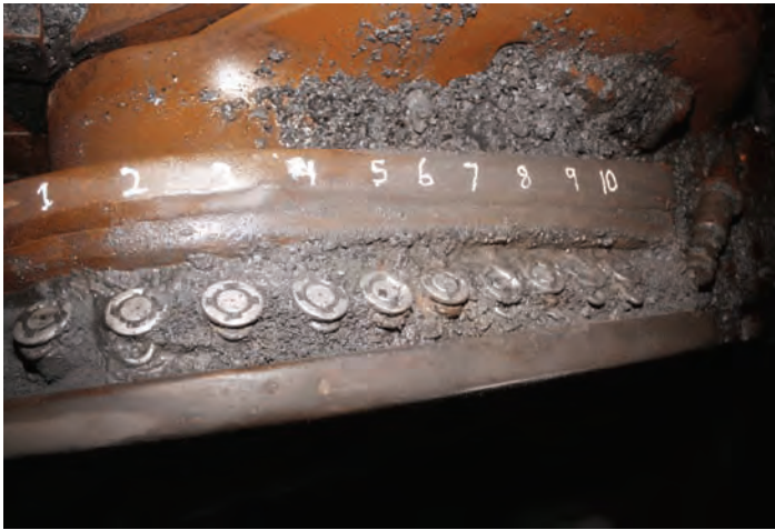
Headgate ranging arm sprays on the UBB longwall. Five of the ten sprays were plugged and did not work.
