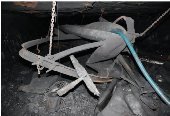
Tailgate 22 section belt and belt structure bent, twisted from forces of explosion.
