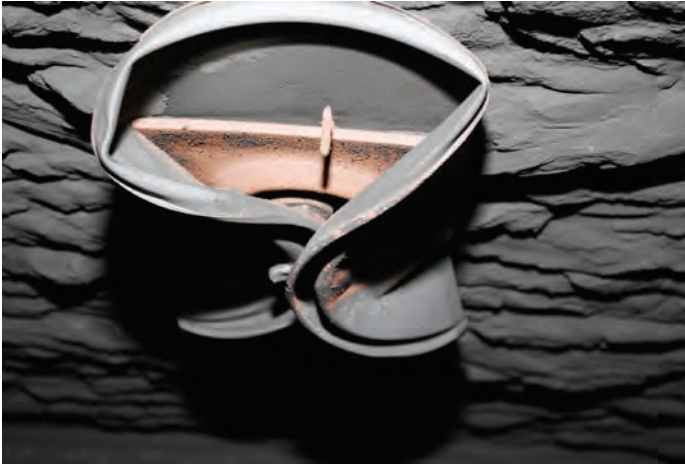
Roof bolt plate bent from initial path (left side) and secondary path (right side) of explosion.
