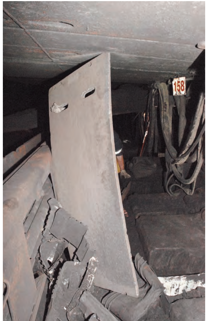
Photo 10. Tail drive assembly lid wedged between top of longwall shield and toes of shield at Shield #158.
