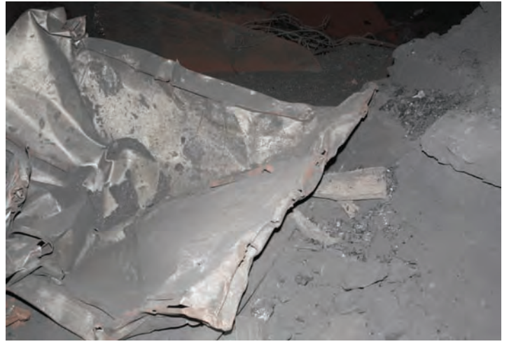
Photo 8. Airlock door blown from hinges and twisted, one block outby Tailgate 22 belt dump.
