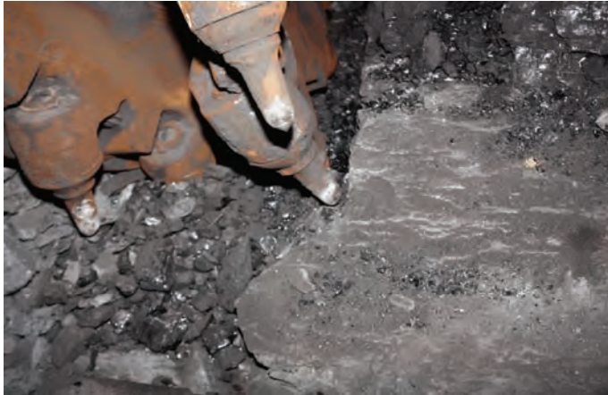
Photo 1. The longwall taildrum bits in a cut-out at the tail. The UMWA believes sparking from this area caused an initial methane ignition, which then grew into a coal dust explosion.
