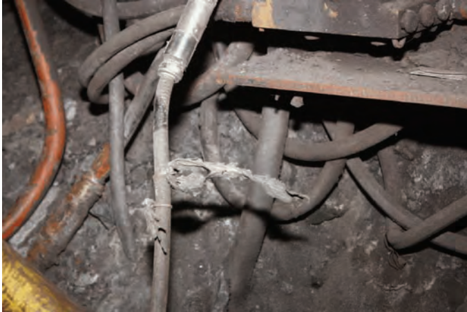
Melted canvas and plastic ties on air hose where canvas was used to direct airflow onto methane sensor on the longwall.
