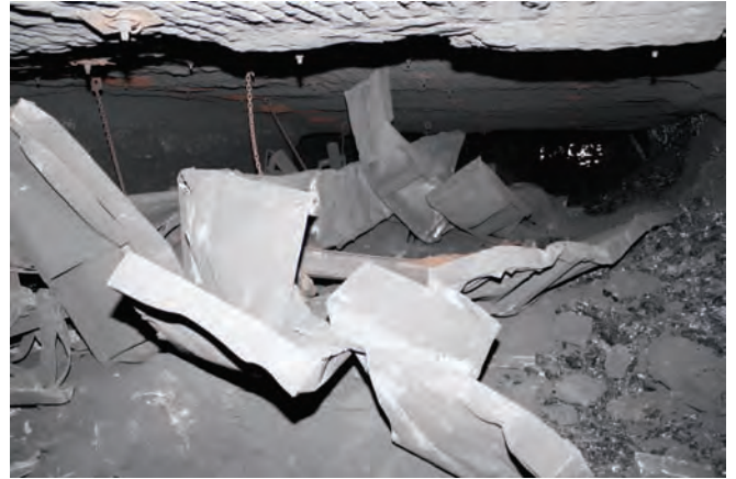
Photo 2. Steel overcast cover panels twisted and crumpled at #1 Crosscut in the Tailgate 22 Section.
