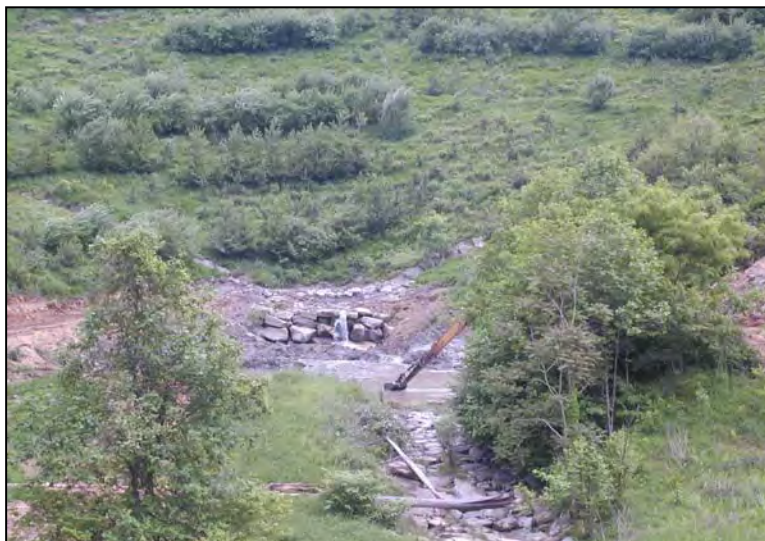
Figure 6. Close-up view of pond cleanout activities. Note the flow coming out of the toe of the hollowfill. The conductivity in receiving stream was 1235 \mu\text{S}/\text{cm} .
