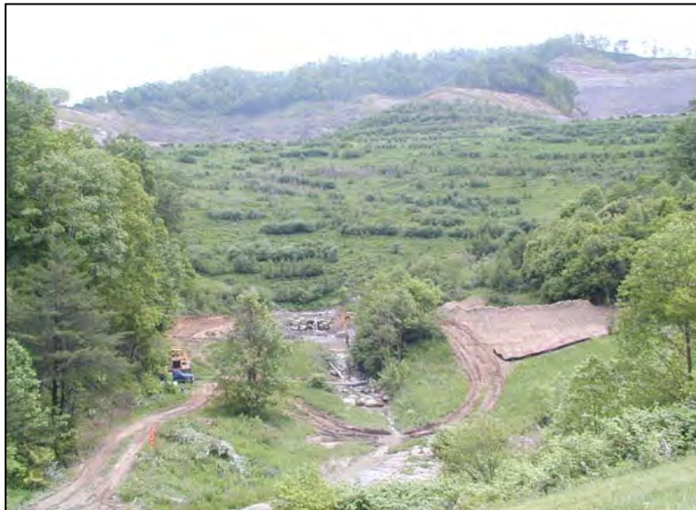
Figure 5. Eastern Kentucky hollowfill setting showing typical worksite for pond cleanout and removal activities.
