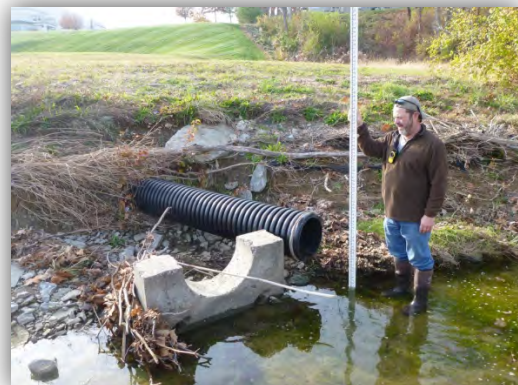
Figure 16-Storm Sewer Infrastructure at Site SFG5.3-DS Compromised by Flow Regime
