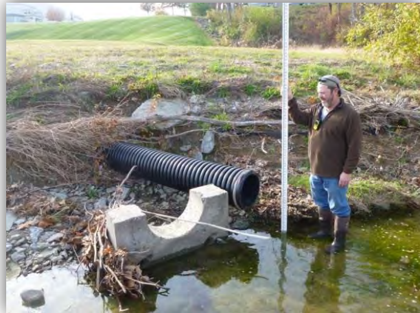
Figure 14: Storm sewer infrastructure at Site SFG 5.3-DS compromised by erosive, urban flow regime
