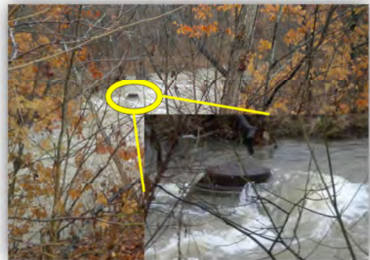
Figure 4-5: Streams widen and destroy public infrastructure
