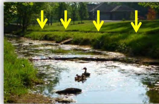
Figure ES-6: SFG 5.3-UNT 0.1 tension crack bank failure
