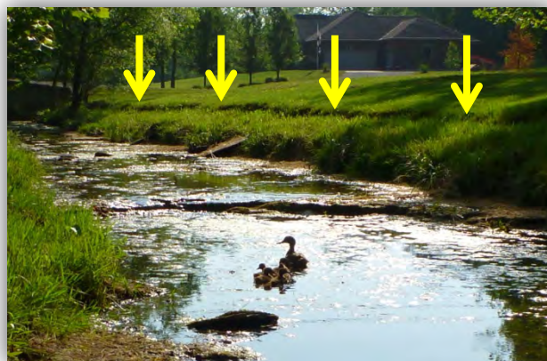
Figure 19-SFG 5.3-UNT 0.1 Tension Crack Bank Failure
