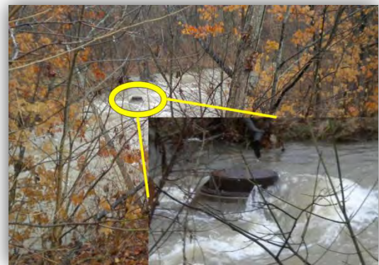
Figure 8: Streams widen and destroy public infrastructure
