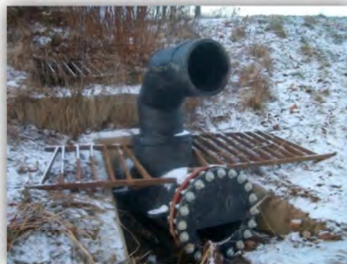
Figure 5-12: Detention basin retrofit outlet structure with bypass, located at Toyota pilot project in Burlington, KY (Photo by Rajib Sinha)
