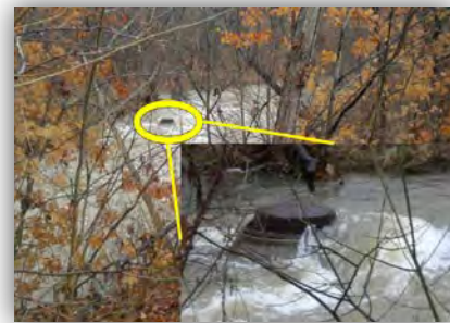
Figure 10-Streams Widen and Destroy Public Infrastructure
