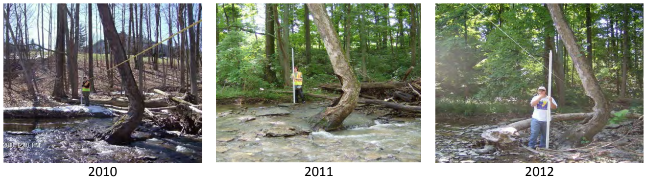
Figure 20-Erosive Flows at GPC 17.1-UNT 0.1 Transport Large Woody Debris and Damage Tree
