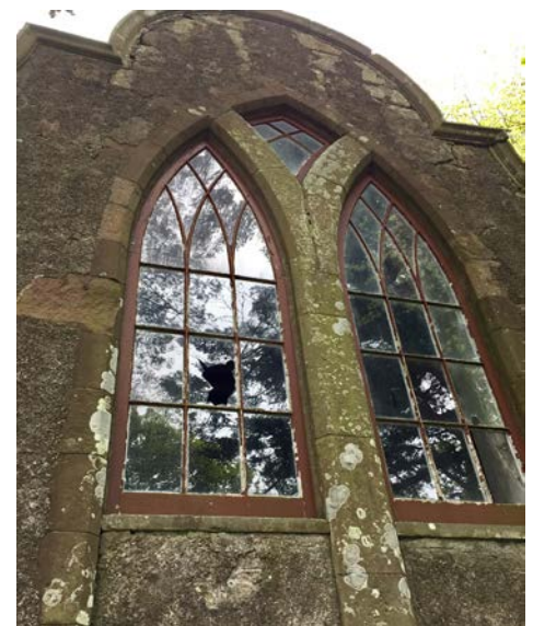
Windows in need of repair at Baird/Barclay Houff at Ury
