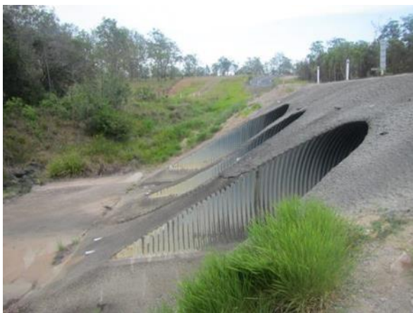
Figure 2.5.5: This road culvert over Island Creek is designed to handle large flows however is lacking 'structure' to facilitate fish passage during high flow events. Structures, such as embedded rocks, provide shelter for fish from the water velocity and also from predation
