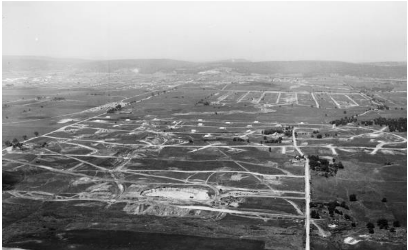
Figure 17: Construction of the Magazine Area, looking north. The Central Grassland is in the middle and the Baraboo Hills are seen in the distance. UW-Madison researchers have conducted grazing experiments with goats on Dairy Forage Research Center lands near the left side of the photo.
