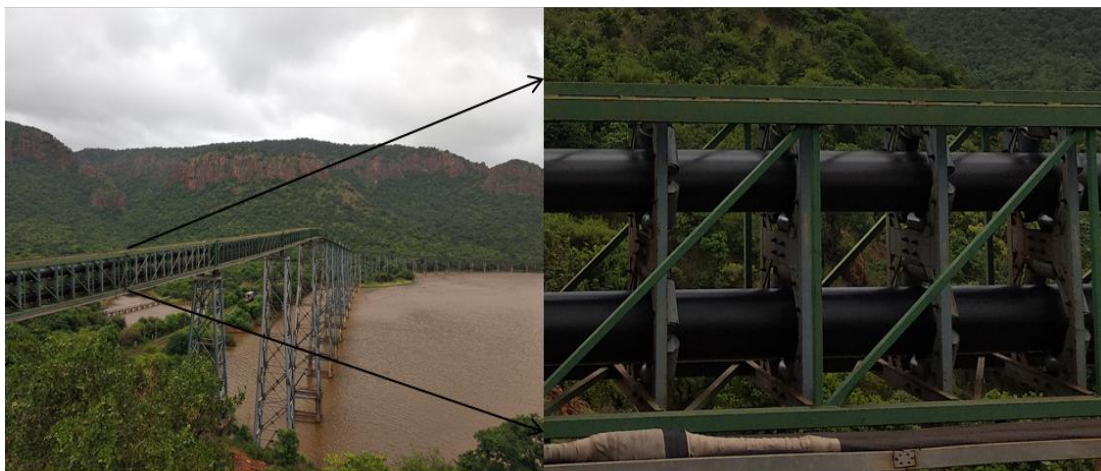
Figure 1.2. Field photograph depiction of Main Pipe Conveyor belt at Narihalla, Sandur, Karnataka.
