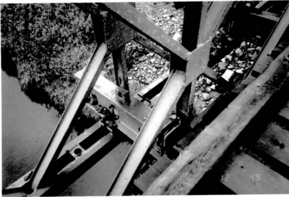
7. Km. 30. Rowlinson Creek Bridge - missing transom clamp
