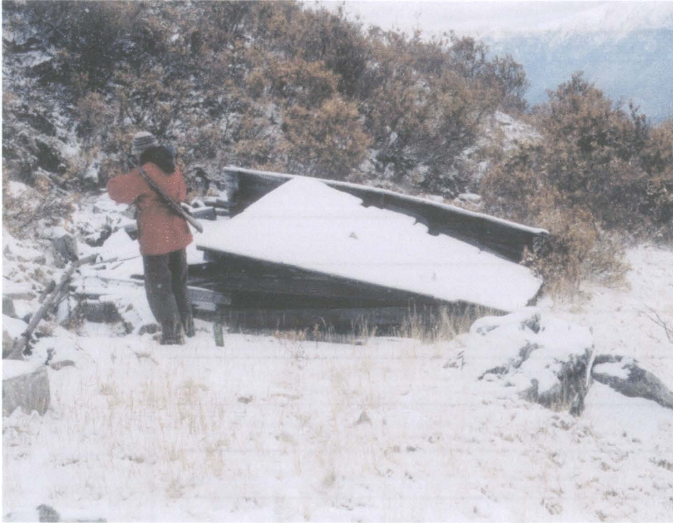
Photo: collapsed building, pipe and steel at the lower adit.
