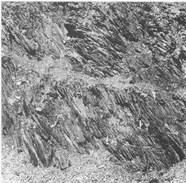
Figure 37. Weathered Harpers phyllite associated with environmental geology unit 6. Artificial cuts in this unit are very susceptible to erosion and weather into piles of slaty talus.
