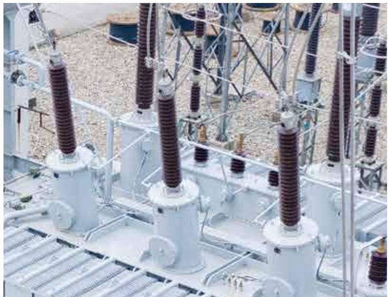
Fig.: High voltage transformer bushing
