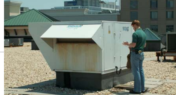
A CEEE researcher performs an energy audit of a rooftop heating and cooling system.
