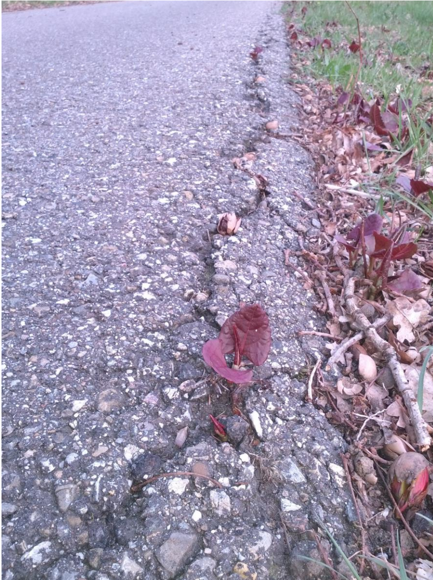
Figure 3.6 Bohemian knotweed penetrating a crack in the asphalt (Ruud Beringen).
