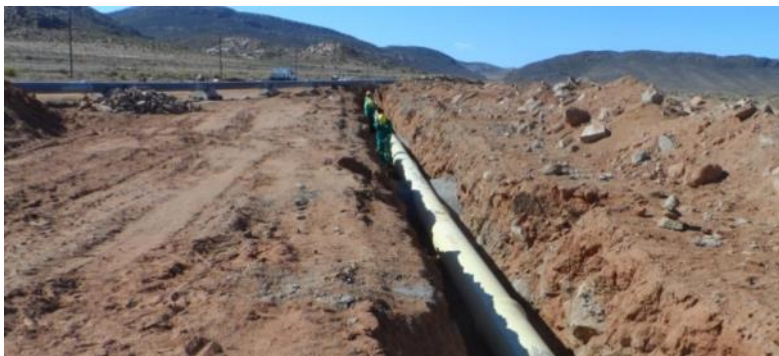
Photo 1: Typical underground construction method (albeit for a much larger pipe), note construction footprint.
