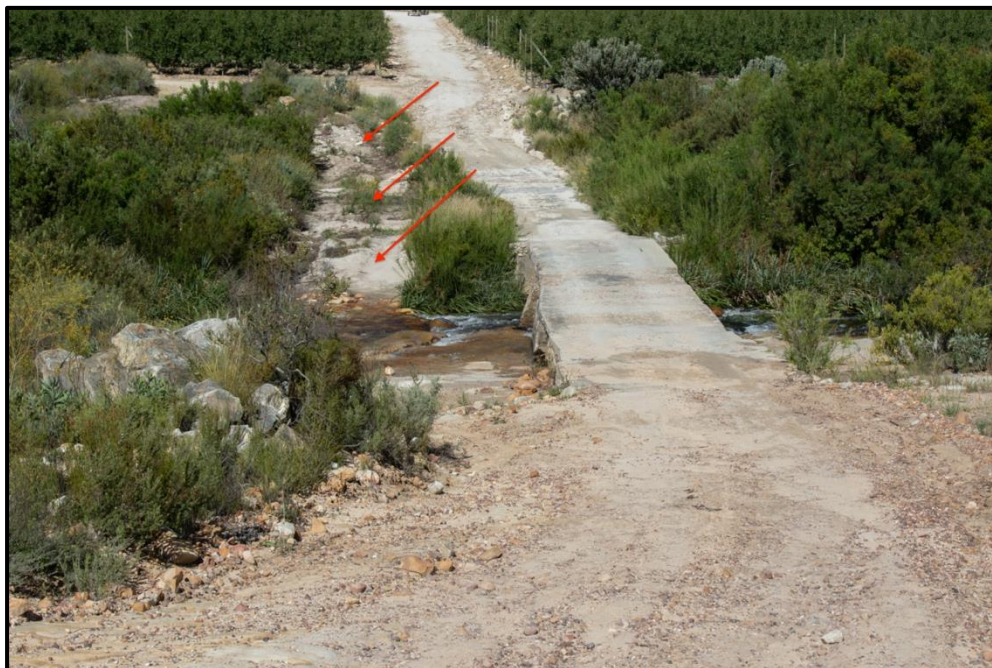
Figure 16. The existing bridge over the Olifants River with disturbance of the riparian zone shown by the red arrows.
