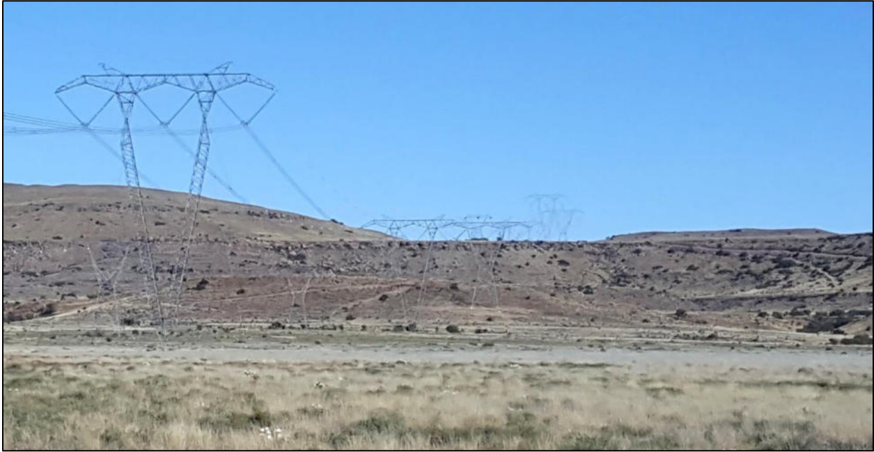
Figure 6. The Gamma 400kV Gridline Corridor also includes rocky hills which correspond with the Upper Karoo Hardeveld vegetation type and are more likely to harbour plant species of conservation concern than the open plains, although no such species were observed in the corridor during the current assessment.
