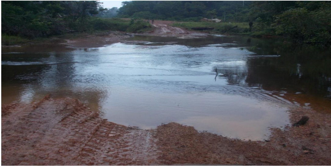
Figure 8: Photograph showing the overtopped state of the Kumung-Kumung Bridge, KPR
