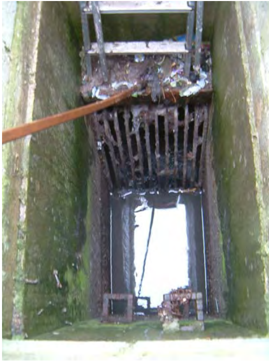
Photo 2.1 Inlet Screening on western network
