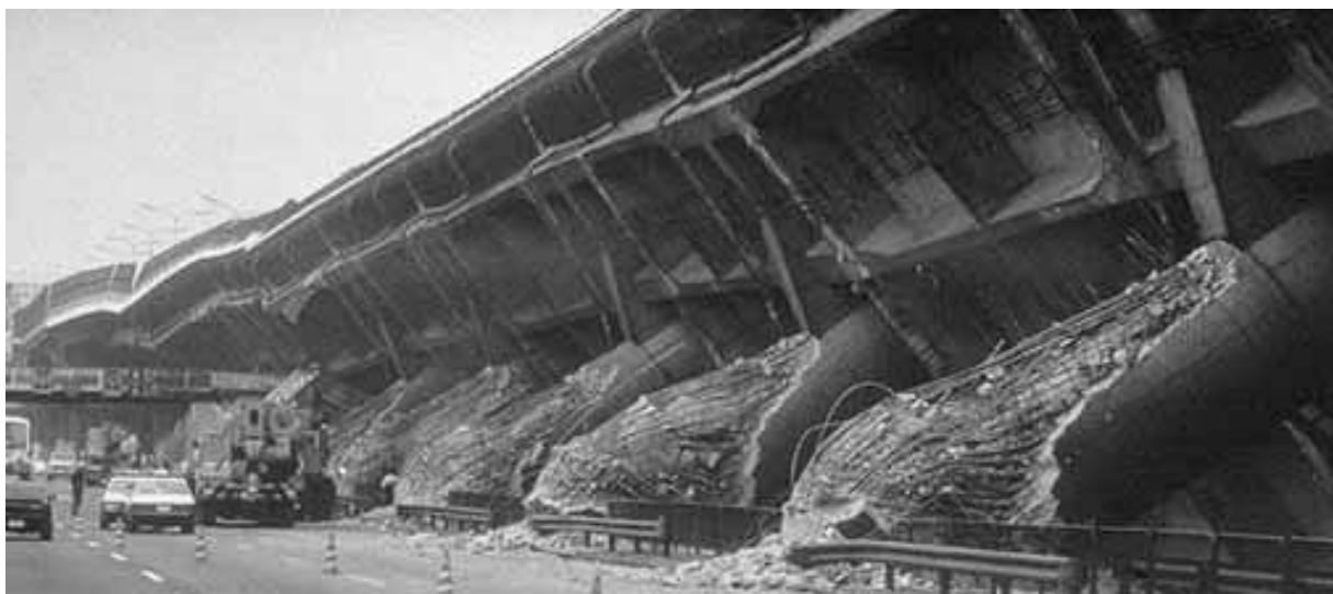
Figure 3. Hanshin Expressway elevated road, Japan (1995)
