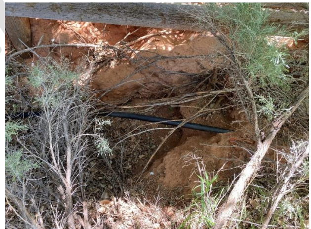
Figure 15: Incised channel forming near enclosure fence at Sykes Spring is exposing pipe infrastructure that was installed to convey water down spring.
