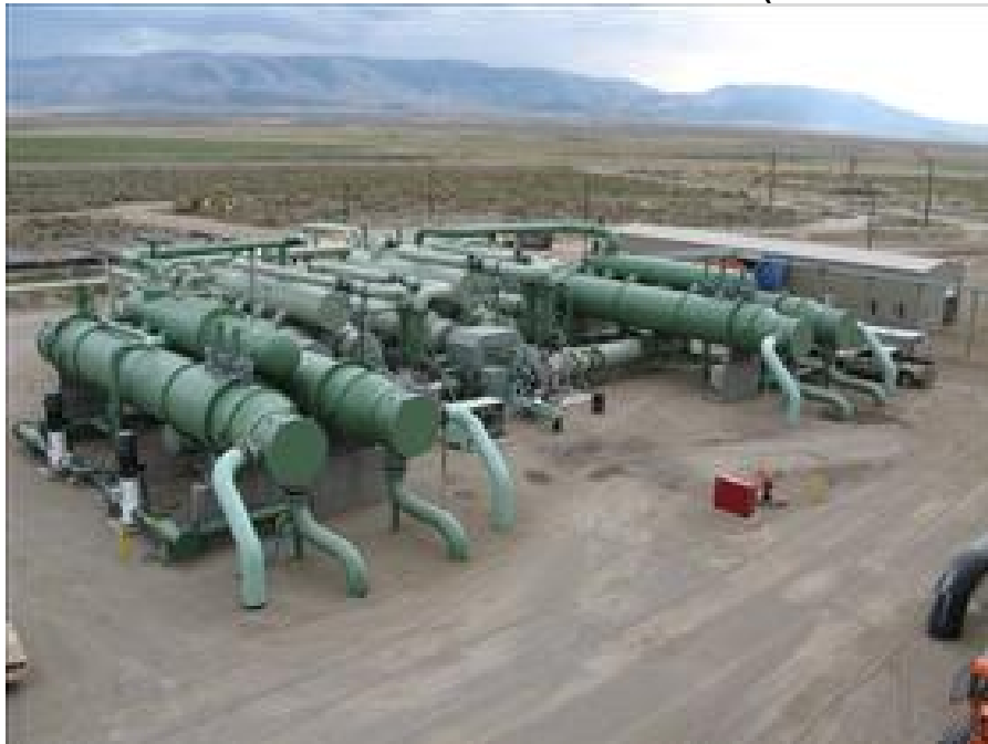
Figure 3. 10-MW Power Plant at US Geothermal Inc's Raft River Site (from US Geothermal Website)
