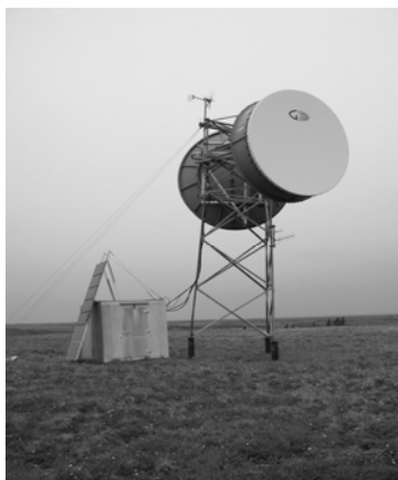
Photo 3.14. Iliamna West Block Communication Site
