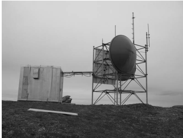
Photo 3.13. Bristol Bay Cellular Partnership Communications Site
