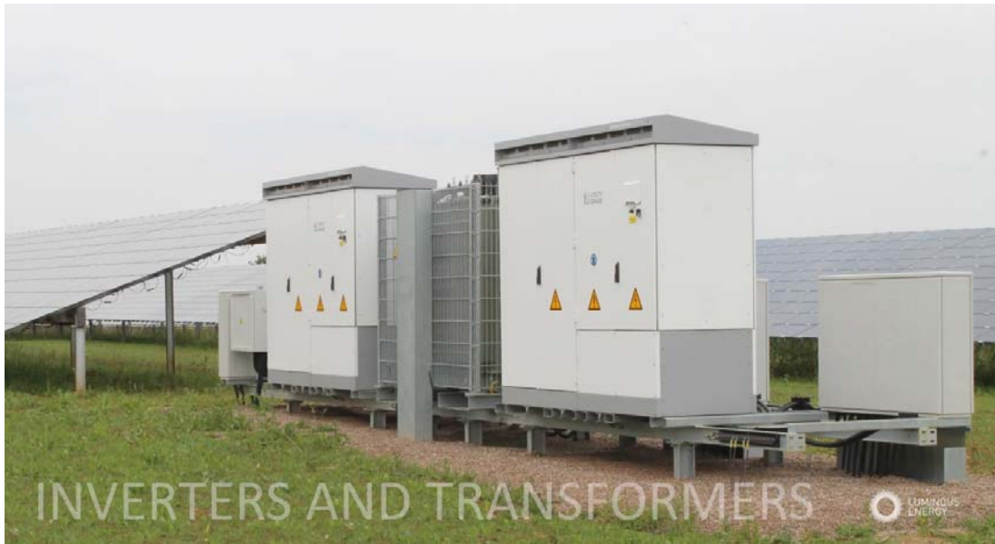
Figure 6 Photographs of a Typical Power Conversion Station/Inverter
