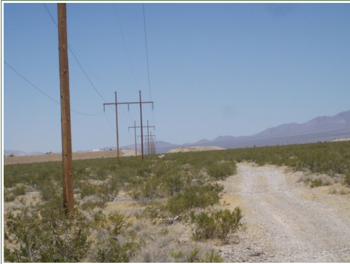
Photo 1. Existing H Frame near Pahrump. Note the existing wires on the top ends of vertical poles.
