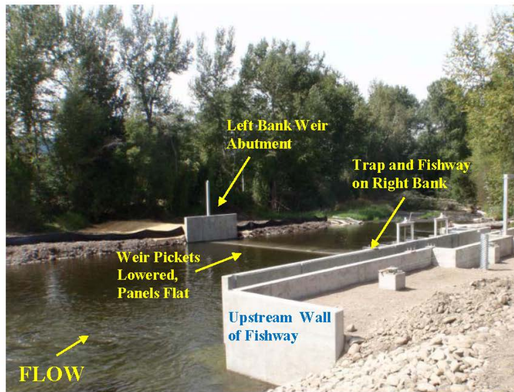
Figure 2-2. Photographs of the Similar Weir and Fishway/Trap in Lostine, Oregon (Recently constructed facility, immediately post-construction, plantings not yet established along banks). Photos show both operational and non-operational periods with weir raised and lowered. Top photo shows weir raised, bottom photo shows weir lowered. The fish weir on Lolo Creek would look similar to this structure.
