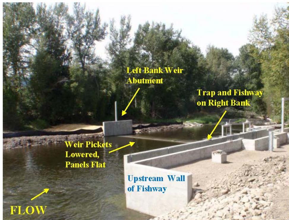
Figure 5. Photographs of the Lostine River Satellite Facility Weir and Fishway/Trap in Lostine, Oregon (immediately post-construction, plantings not yet established along banks).
