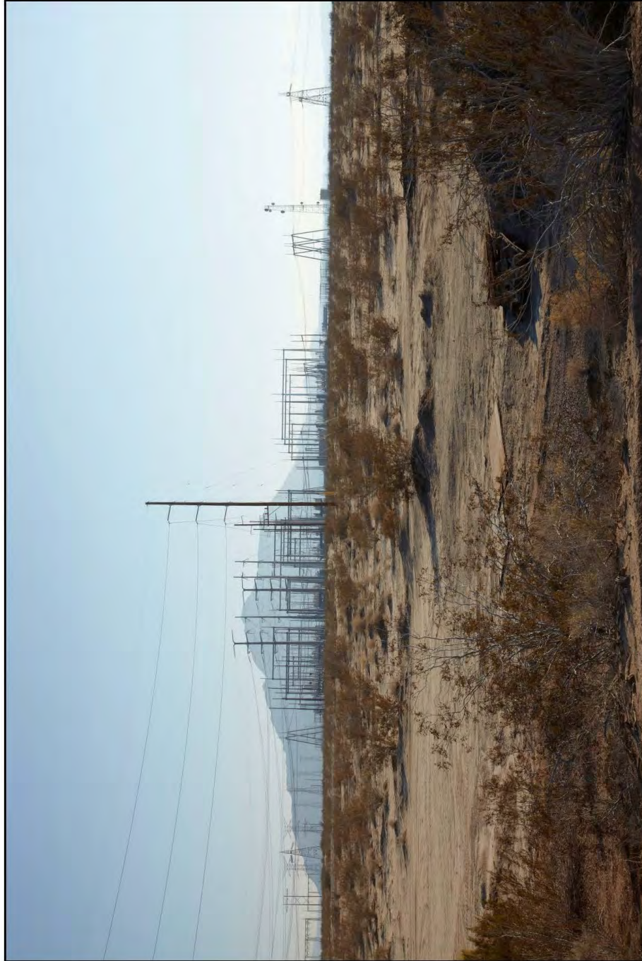
Figure 3-5 Existing View of Alternative 3 Gen-Tie Route On BLM Land Looking South Towards Imperial Valley Substation
