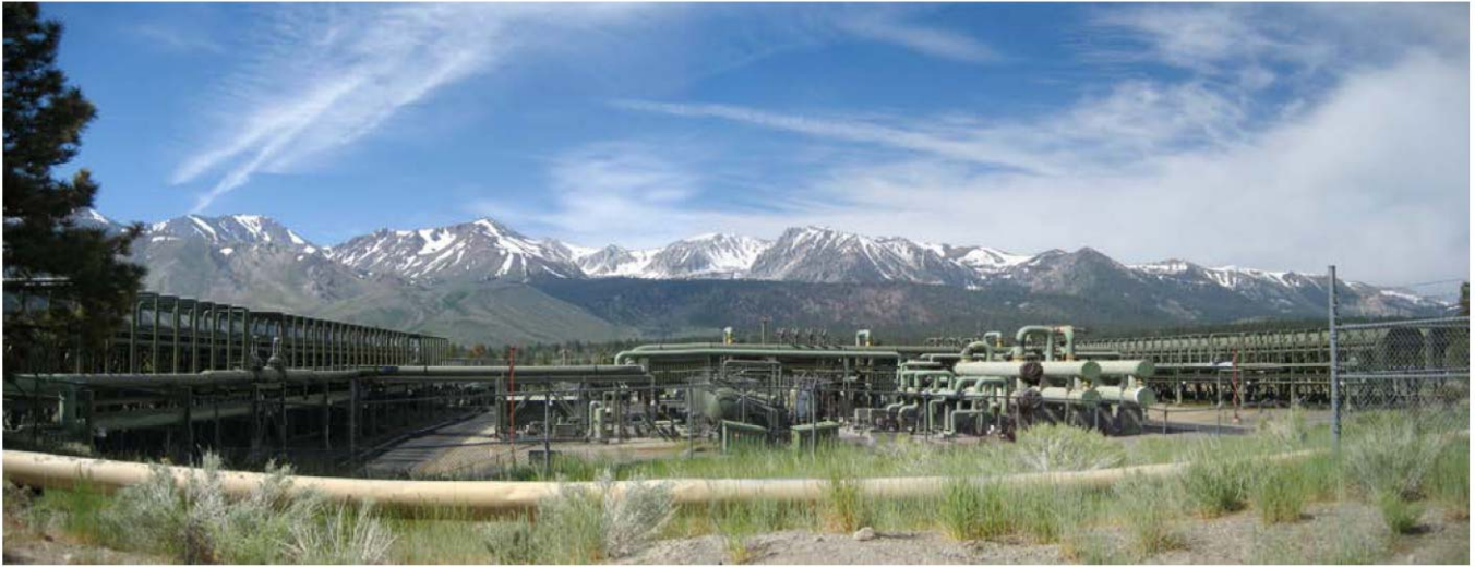
Photo 1 Existing geothermal power plant near junction of Highway 395 and SR 203, looking west
