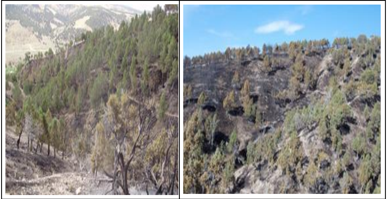
Figure K-14. Mechanical Treatments with Chainsaw. Units 1, 2, 3 were all thinned with chainsaws and Unit 2 & 3 were piled and burned. Unit 3 had two entries of thinning and the leave trees were limbed 3-4 foot high.
