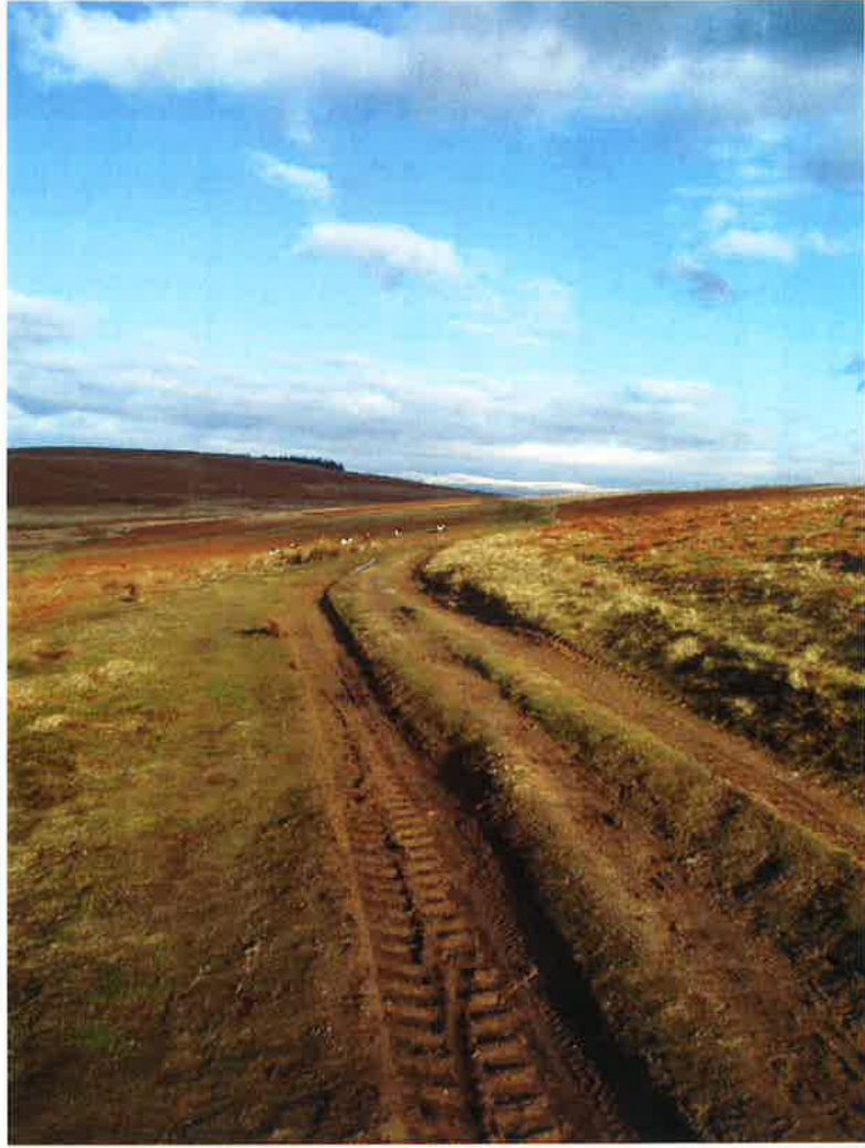
Plate 11: Deep wheel rut damage to the Askham Fell Bridle way
