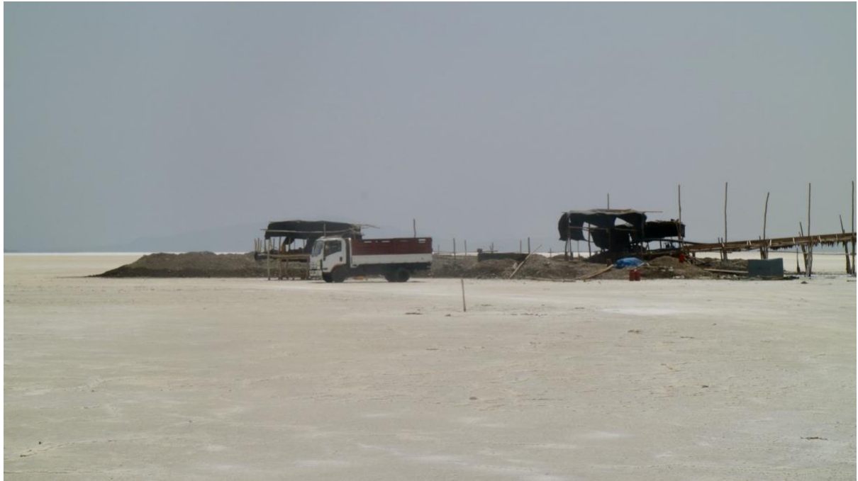
Image 19: Construction site to establish large salt works in the ‘Afar Depression the salt flats (photo: TJFT, August 2018)
