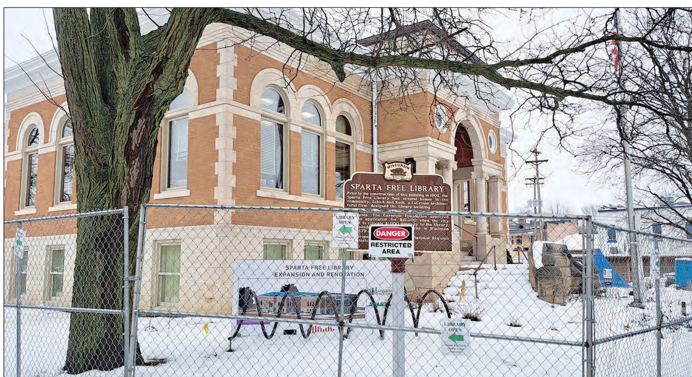
The Sparta Free Library is currently in the process of building an addition on its eastern perimeter, as well as remodeling the Carnegie structure, in which it resides. Director, Michelle Tryggestad, states that entire project will be completed by next January. The structural steel will arrive on site this week, and it is expected to be up within a short time. Herald photo by Benny Mailman.
