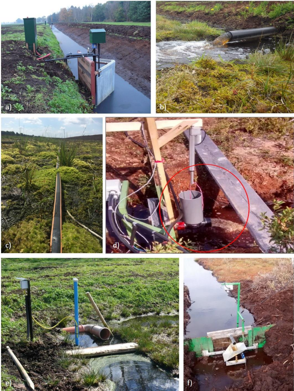
Figure 4. Water management components for Sphagnum farming sites: a) electric pump (Rastede); b) inlet into the irrigation ditches (Rastede); c) drip irrigation (Drenth); d) 'adjustable ditch' with an outlet (Shippagan 2); e) outlet with a data logger (Rastede); f) outlet (Saint-Modeste). Photos: a) and e) Sabine Wichmann, b) Greta Gaudig, c) Dorothea Rammes, d) and f) Peatland Ecology Research Group.
