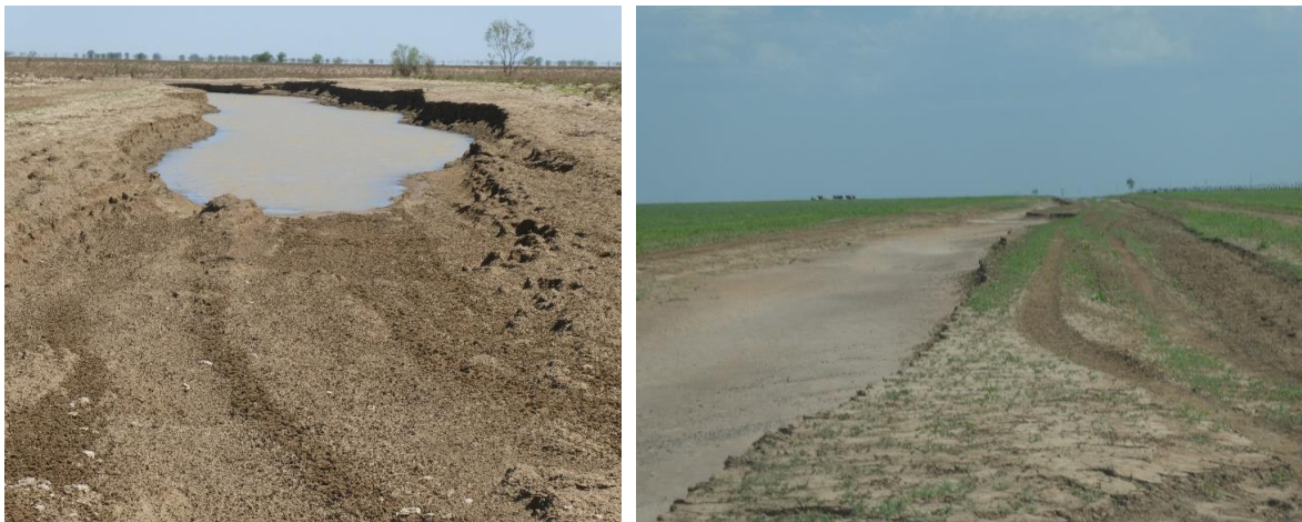
Figure 36a, 36b. Washed out Council maintained main roads (a) Punchbowl to Nelia road NE of Julia Creek, and (b) Gilliat to McKinlay road SW of Julia Creek.
