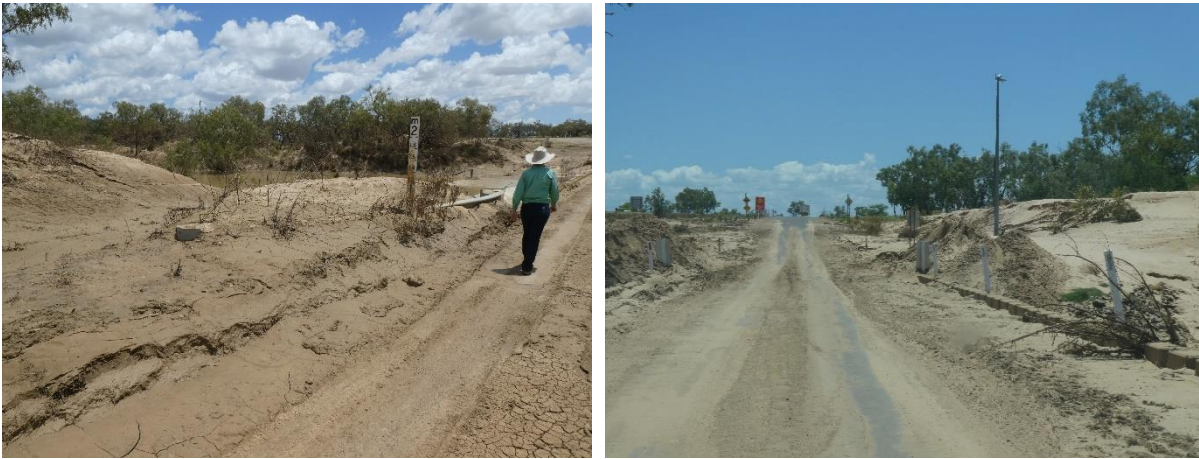
Figure 37a, 37b. Deep silt deposition on Council maintained main roads, causeways and bridges north of Julia Creek.
