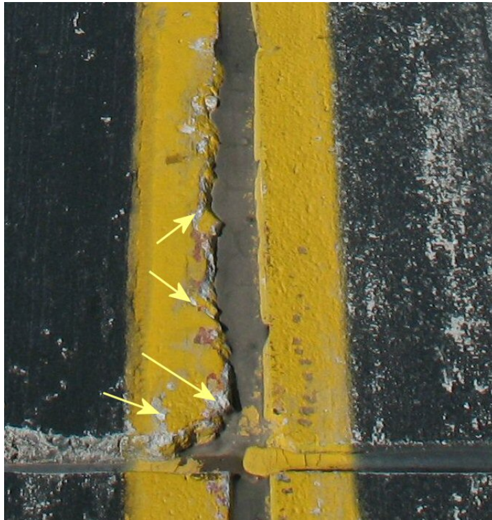
Figure 57. Aggregate suspected of being nondurable in a zone of heavy raveling.
