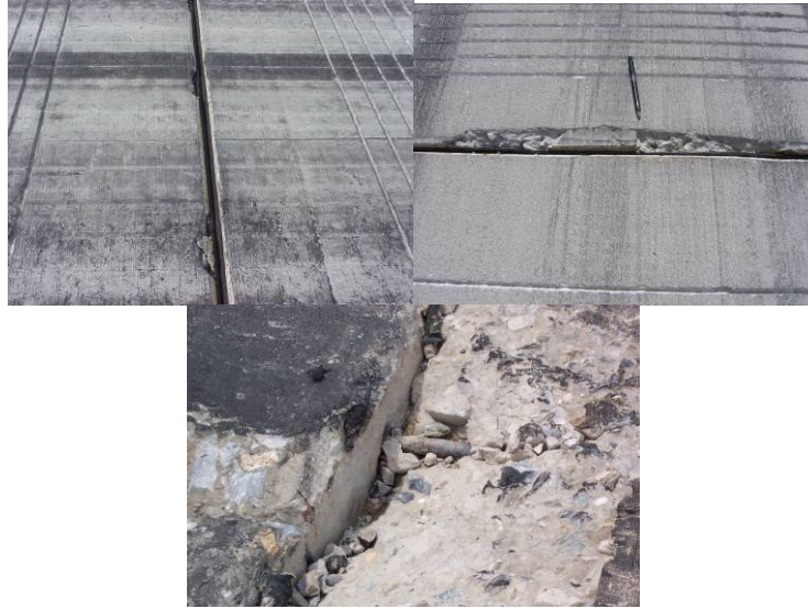
Figure 1. Examples of runway joint spalling: (top left) low-severity spalling, Elmendorf AFB; (top right) medium-severity spalling, Offutt AFB; (bottom) high-severity spalling, Bagram AB
