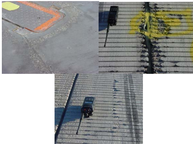
Figure 3. Examples of snowplow damage to USAF airfield pavements: (top left) scraping around raised obstacle; (top right) inexperienced operator damaged centerline, compounded by improper grooving pattern passing through crowned centerline; (bottom) pavement grade change outside of smoothness tolerances resulting in dragging of blade tip of snow-clearing equipment.
