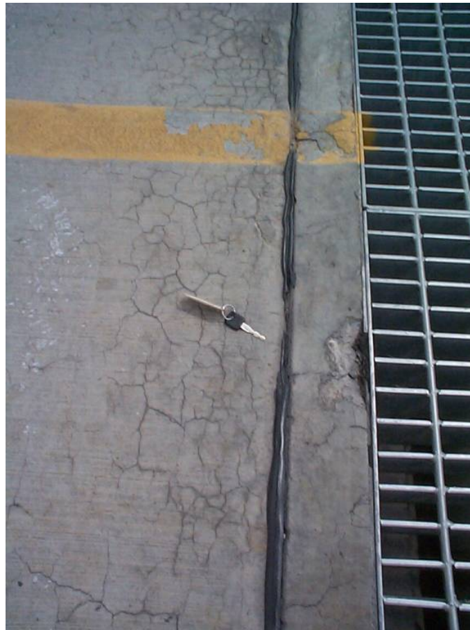
Figure 10. Example of spalling from alkali-silica reaction compressing expansion joint causing spalling at trench drain, Holloman AFB, NM.
