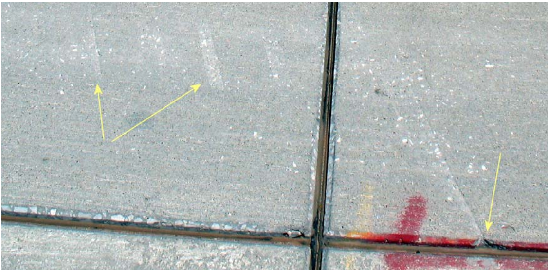
Figure 59. Scars that appear to result from snowplow abrasion, along with damage to the joint (lower right).
