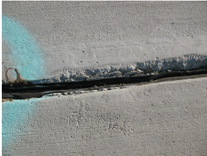
Figure 52. Expansion joint on south side of RW centerline at STA 39+44. Runway slab is to the top.
