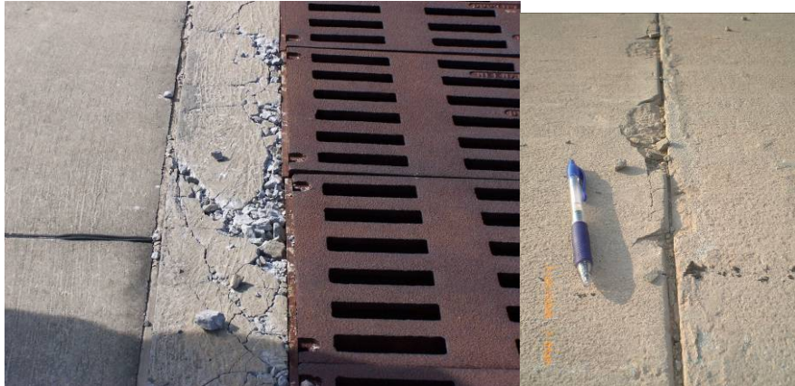
Figure 5. Examples of spalling from volume change restraint: (left) expansion joint material does not extend full depth of pavement, so concrete pavement movement causes spalling at the trench drain, Hurlbert AFB, Florida; (right) debris-clogged joints cannot accommodate temperature-induced movement in concrete pavement, leading to spalling, Middle Eastern airfield.
