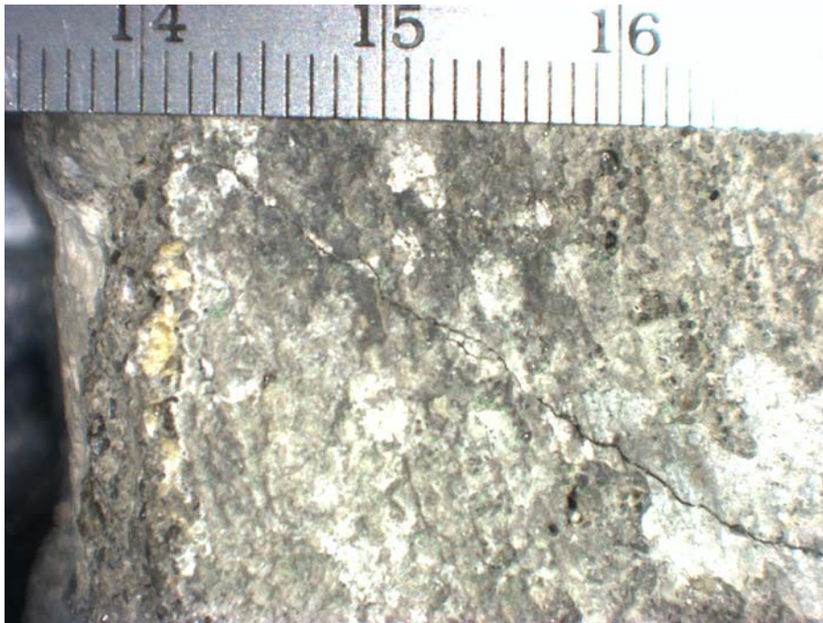
Figure 47. View of a crack on the finished surface of Core 19, taken from TW P. The vertical face to the left is part of an intersecting crack. A piece of nondurable coarse aggregate is visible as the white feature on the vertical face.
