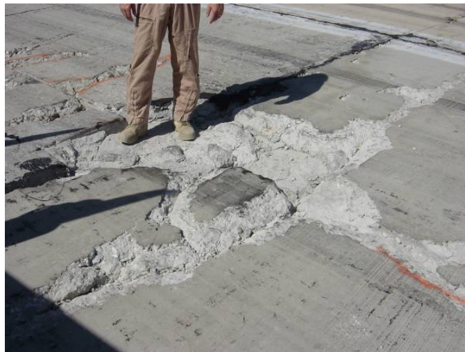
Figure 2. Extensive spalling along joints and cracks caused by excessive structural loading, Bagram AB runway.
