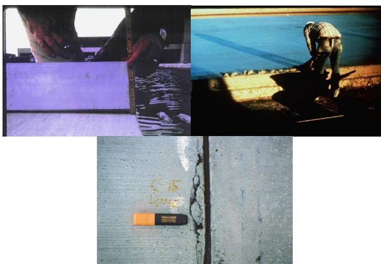
Figure 4. Examples of edge-slump problems with slip-form paving at Travis AFB: (top left) example of edge slump; (top right) attempts to repair by hand; (bottom) failure of edge-slump repairs.
