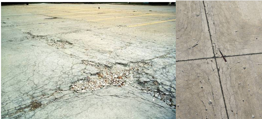
Figure 7. Examples of D-cracking: (left) severe spalling from D-cracking at Grissom AFB, IN; (right) moderate D-cracking with popouts, St. Joe ANG facility, MO.
