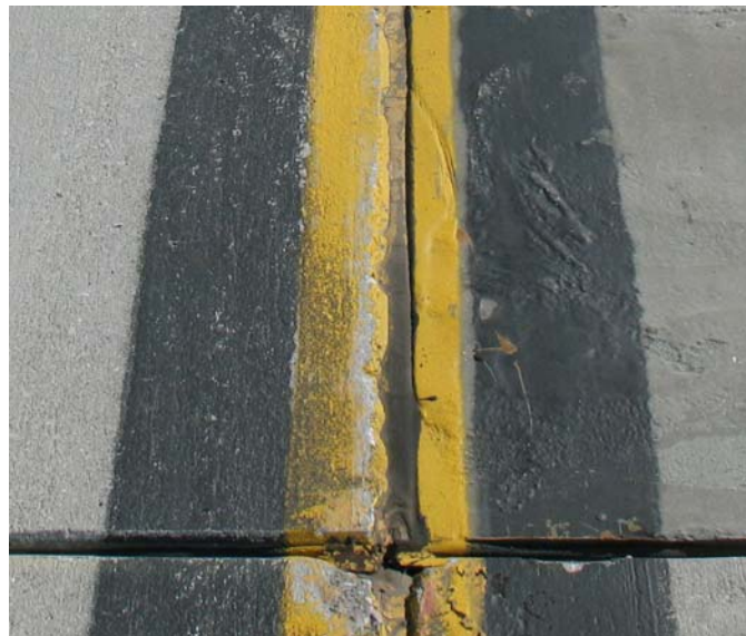
Figure 54. Surface abrasion along a centerline joint.
