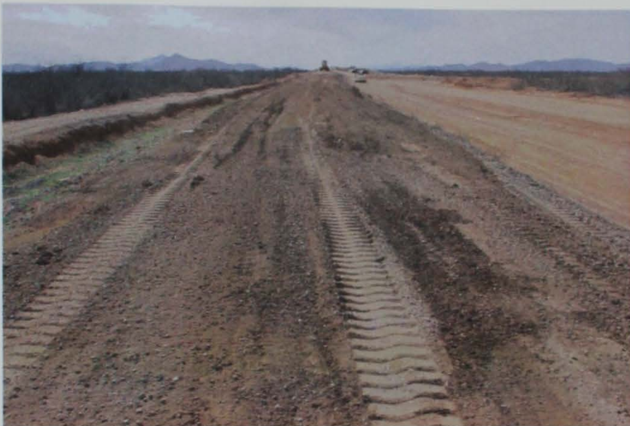
Photo 17. Uncompacted surface on Section 4 with poor product distribution
