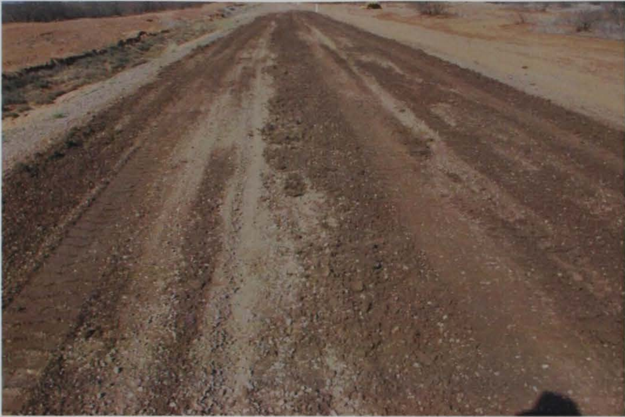
Photo 19. Exposure of untreated areas after grading of surface
