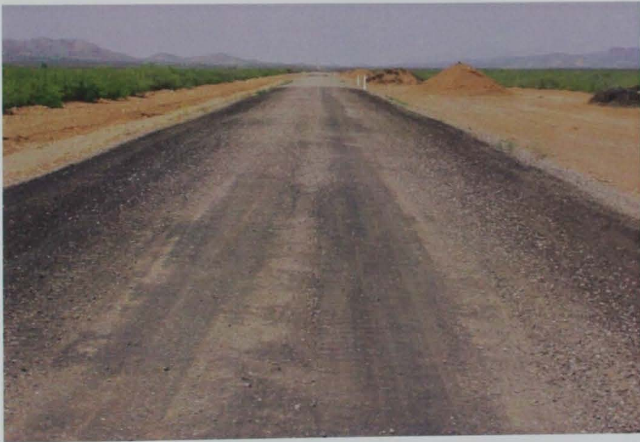
Photo 38. Disturbed surface of asphalt emulsion on Section 23 after 30 days
