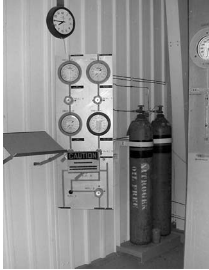
Figure 3. Launcher nitrogen servicing panel and bottles, VAFB Facility #582, 2008 (ERDC-CERL).
