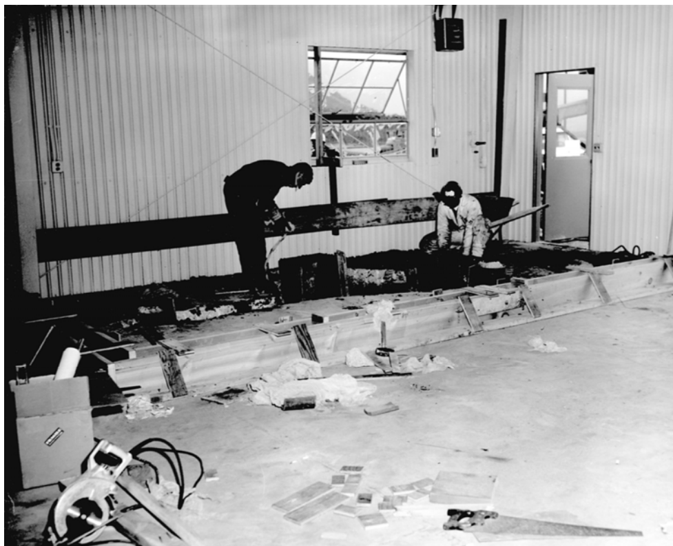
Figure 1. H 2 O 2 system installation in the operations support building, VAFB Facility #582, 5 February 1962 (Official U.S. Navy Photograph).
