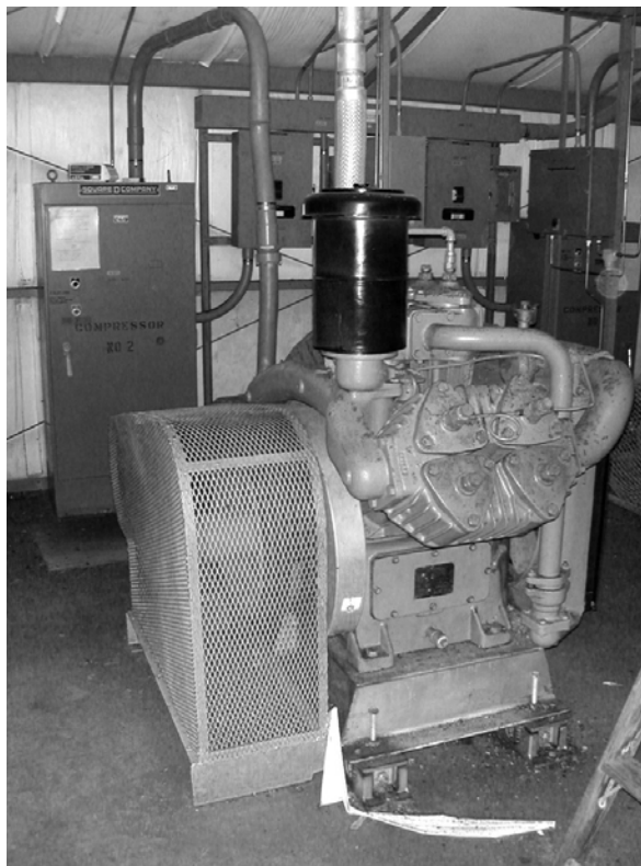
Figure 5. Air compressor in operations support building (VAFB Facility #582) compressor housing addition, 2008 (ERDC-CERL).
