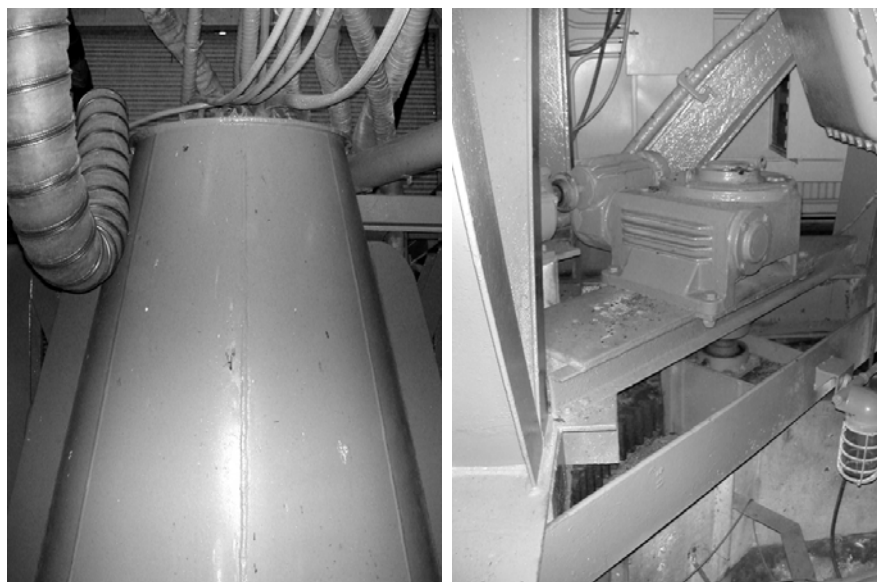
Figure 10. Blast shield assembly (left) and azimuth drive and bearing assemblies (right), VAFB Facility #580, 2008 (ERDC-CERL).
