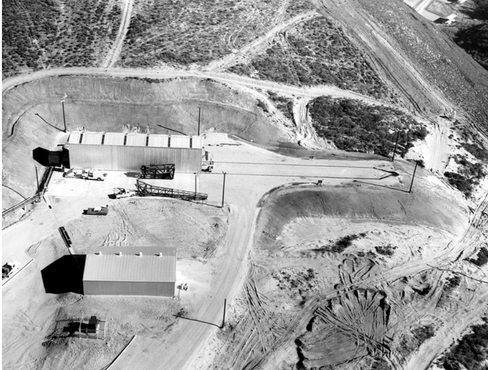
Figure 21. SLC-5 construction showing launcher in two pieces outside mobile shelter, 9 January 1962 (Official USAF Photograph).
