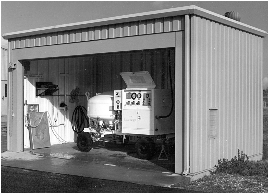
Figure 1. Cryogenic converter unit in Cosmodyne shelter, circa 1981 (Official USAF photograph).
