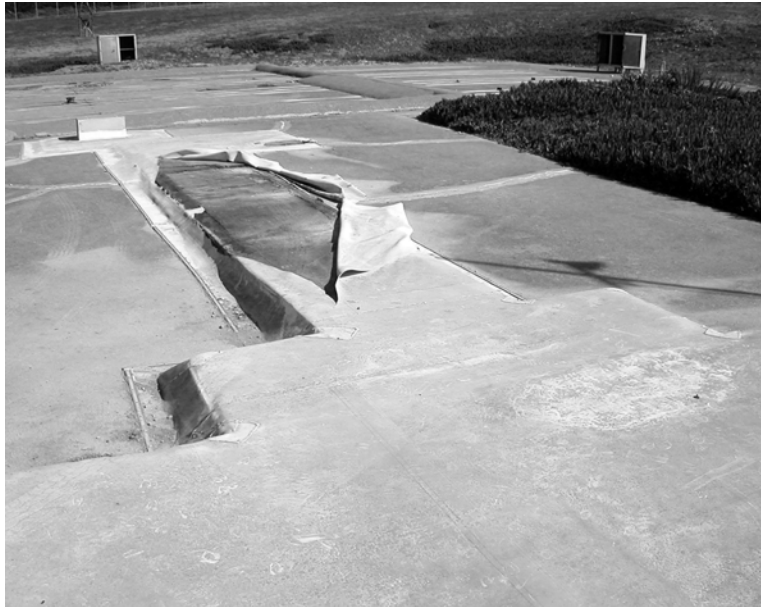
Figure 5. Dual communications/power trench (center) and offset cable vaults (upper left) that distributed power to the pad's TV camera stations, 2008 (ERDC-CERL).
