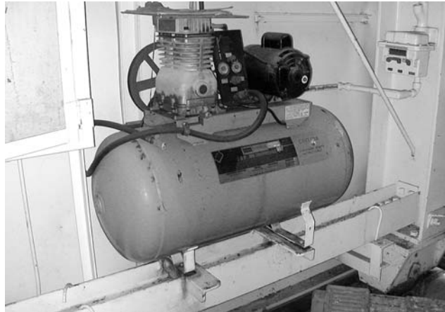
Figure 5. Compressor for inflatable seals, VAFB Facility #580, 2008 (ERDC-CERL).
