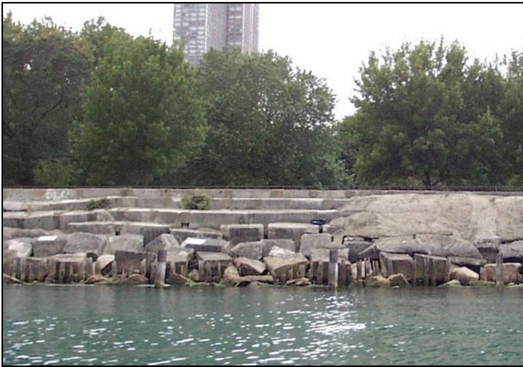
Figure 4. Example of revetment failure along Montrose to Irving reach (photograph courtesy of U.S. Army Engineer District, Chicago).
