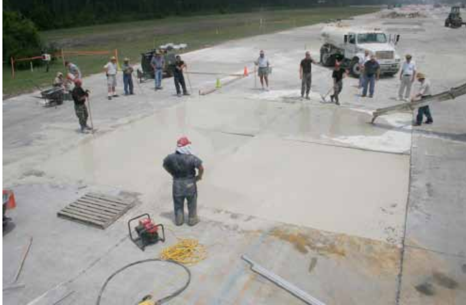
Figure 95. The repair material in Crater 3 is approximately 2 in below the existing pavement surface.
