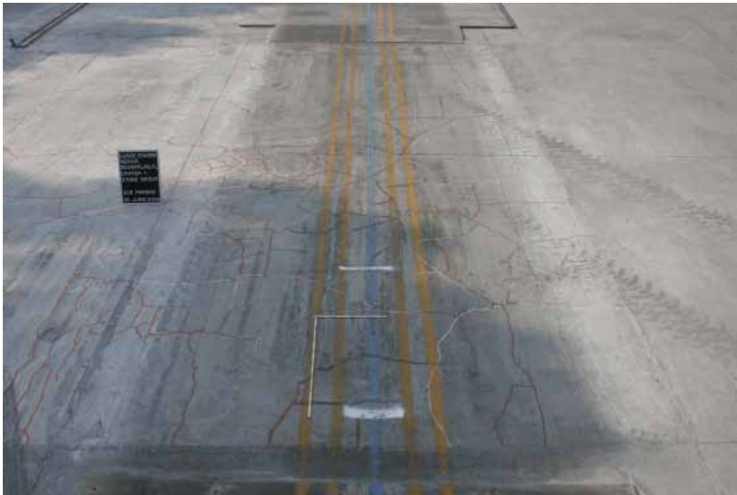
Figure 141. Crater 1 after 528 completed load cart passes.
