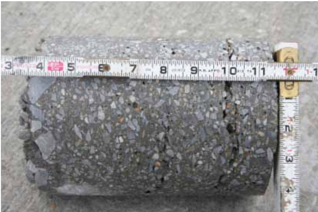
Figure 172. Core 5 from Crater 2 on non-trafficked side of repair, CeraTech Pavemend EX-H showing irregular layers of material separated by void spaces.
