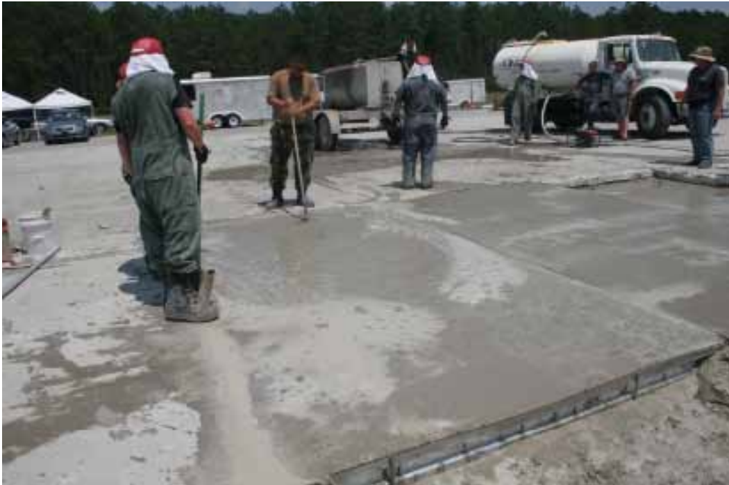
Figure 84. Section 2 of Crater 4 was filled with a portion of the material from Batch 6.
