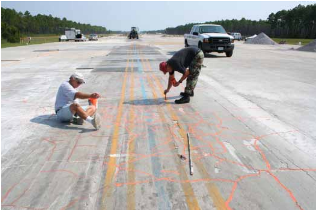
Figure 158. Highlighting cracks on the surface of Crater 1 after 5,008 passes of load cart.
