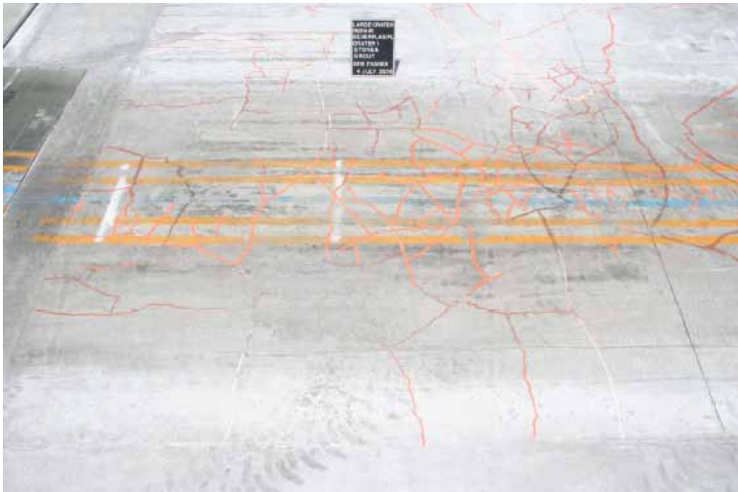
Figure 152. Crater 1 after 2,016 completed load cart passes.
