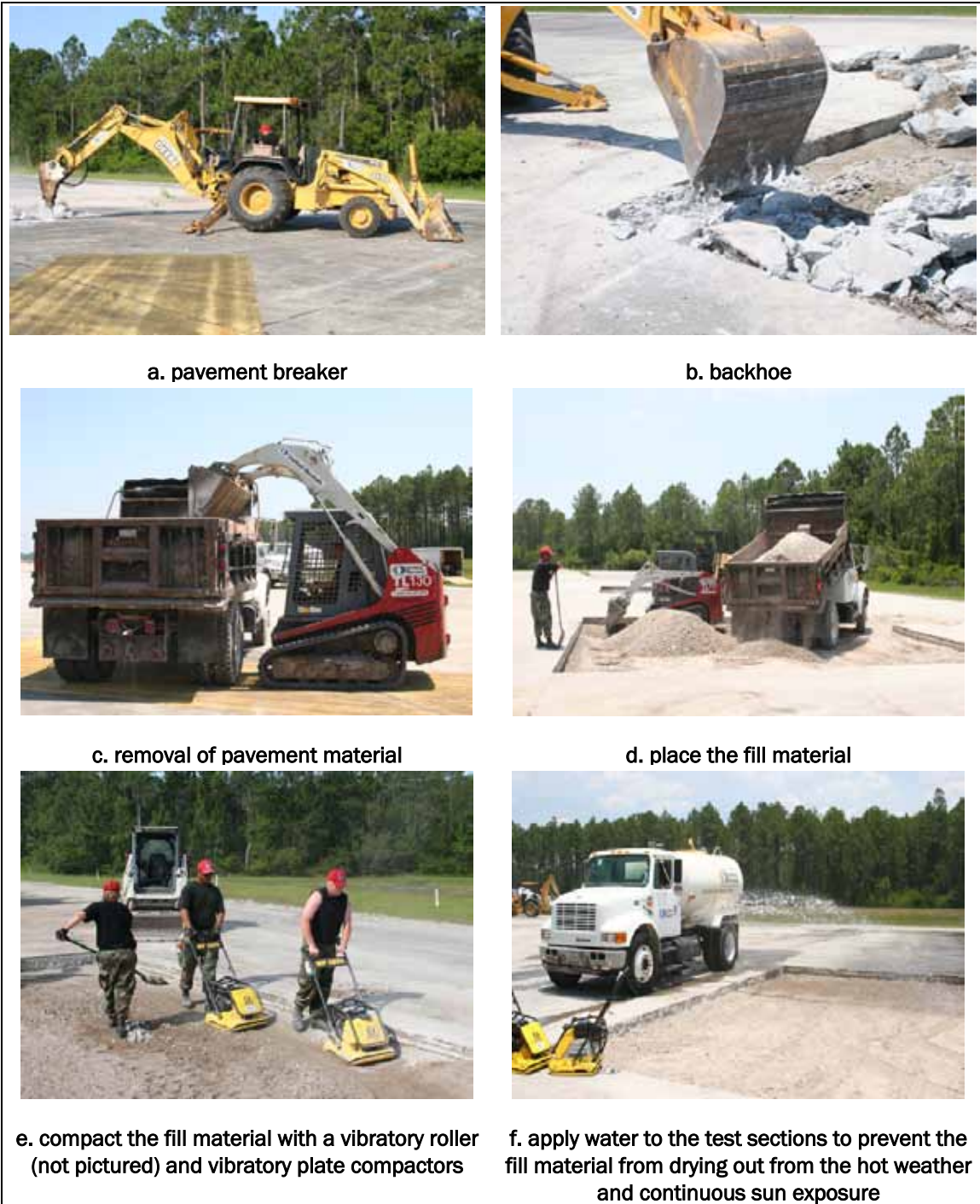
Figure 9. Preparation of the test craters showing the techniques and equipment used to break out and remove existing pavement.
