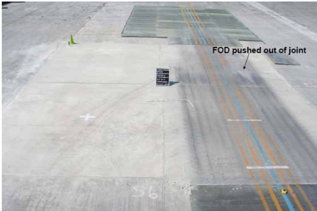
Figure 151. Crater 6 after 1,008 completed load cart passes.
