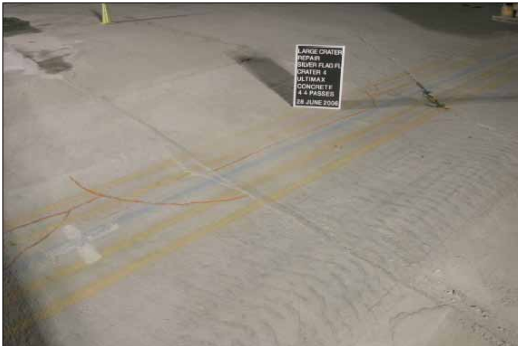
Figure 137. Intersecting cracks after 44 passes in Crater 4.
