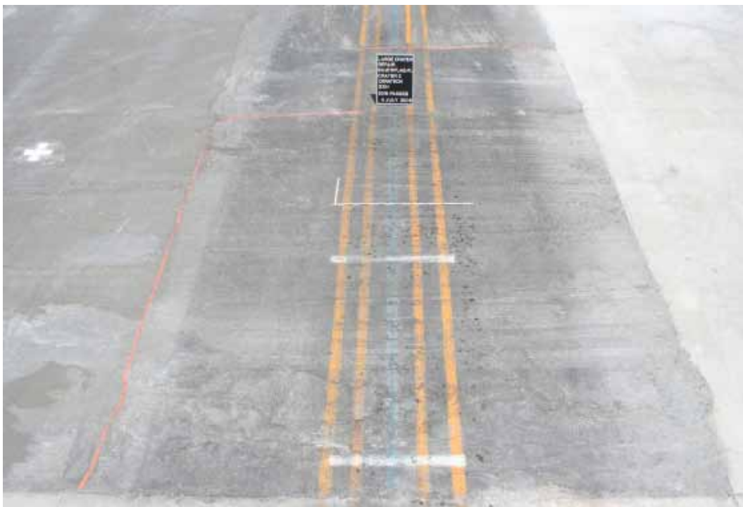
Figure 153. Crater 2 after 2,016 completed load cart passes.
