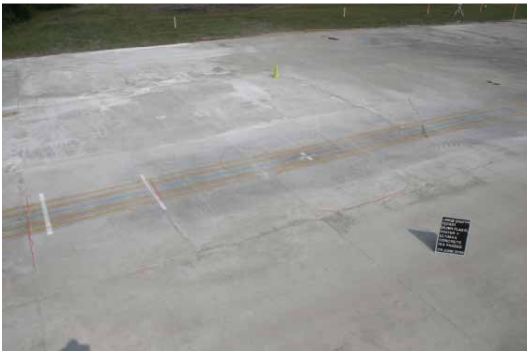
Figure 138. Cracking after 100 passes in Crater 4.
