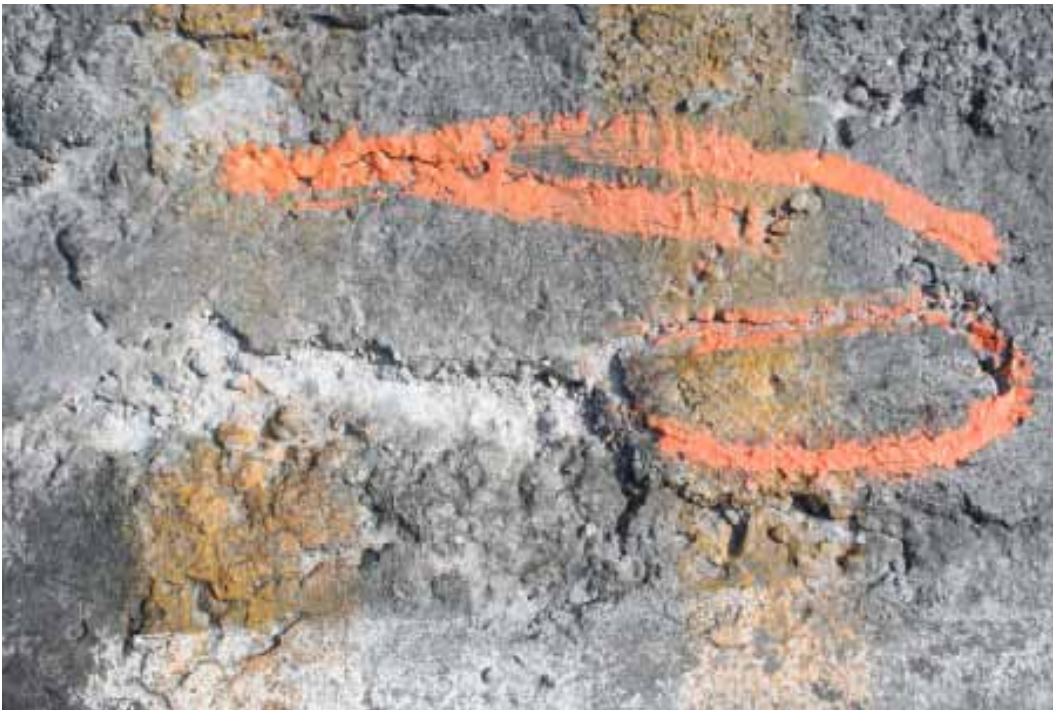
Figure 160. Close up of surface of Crater 2 after 5,008 passes of load cart.
