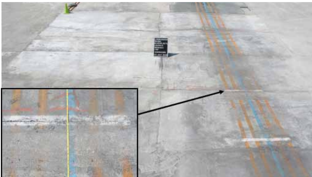
Figure 150. Crater 5 after 1,008 completed load cart passes.
