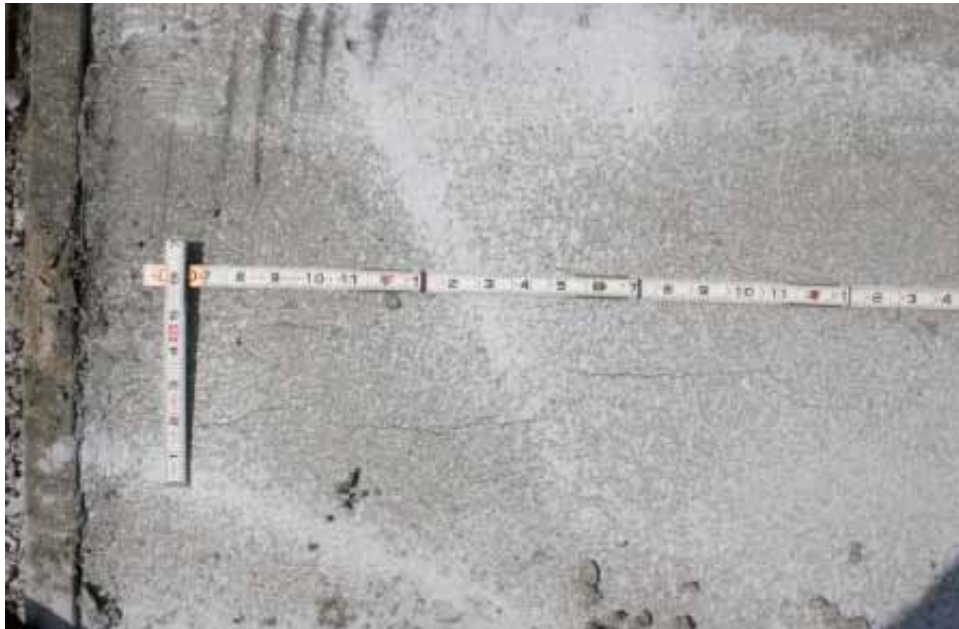
Figure 59. Shrinkage cracks formed in the repaired northwestern quadrant of Crater 5.
