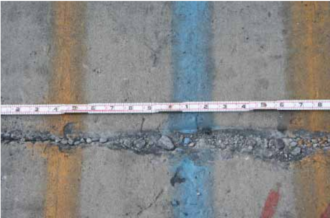
Figure 164. Close-up of joint spall between repaired slabs in traffic lane of Crater 6.
