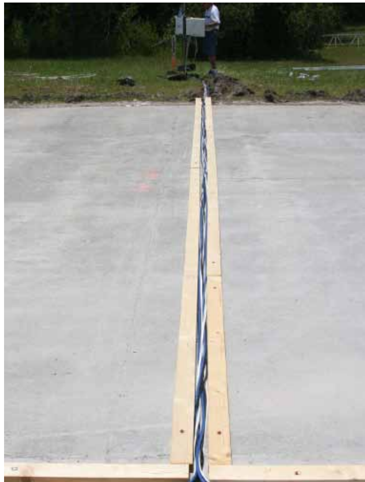
Figure 13. Photograph showing protected instrumentation wires routed to data acquisition system off the runway edge.
