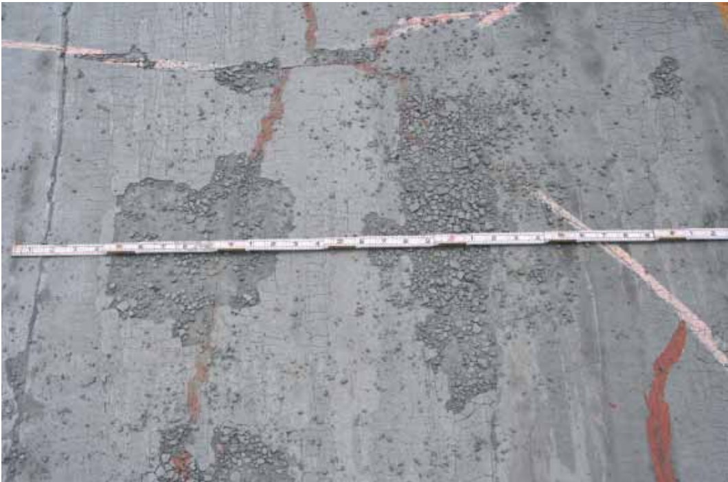
Figure 147. Close-up of FOD, Crater 1 after 1,008 completed load cart passes.
