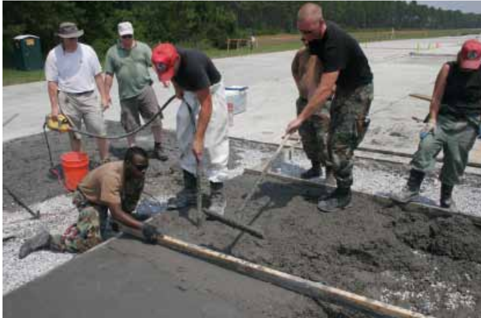
Figure 71. Attempt to finish Batch 11 before it sets up and workability is lost in Crater 2.
