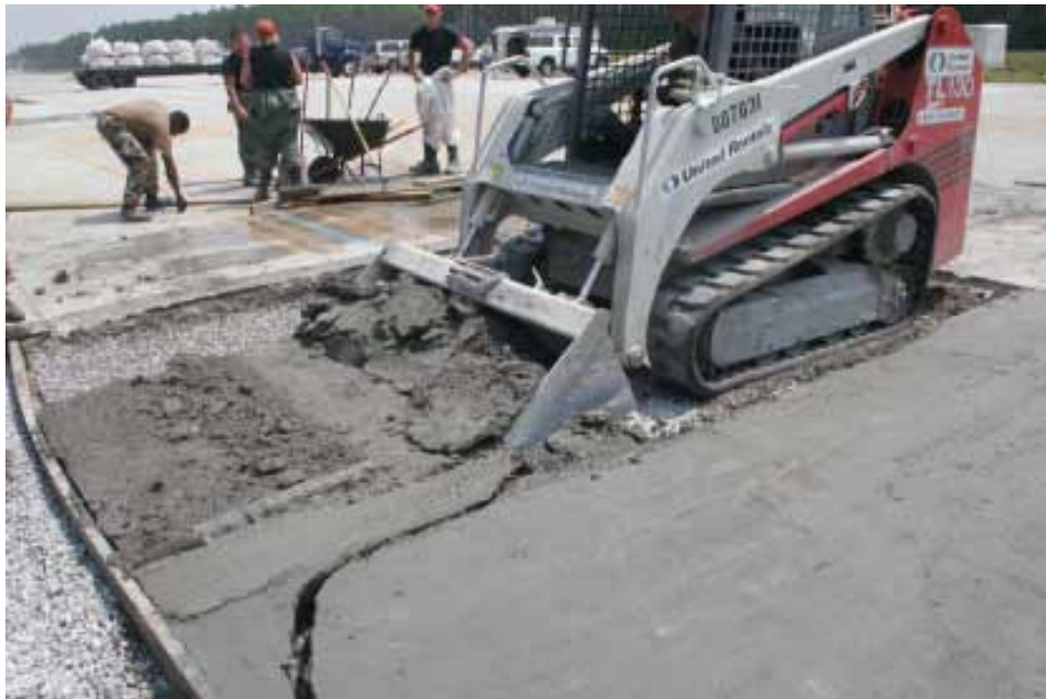
Figure 72. Removal of material from Batch 11 and damage to adjacent section in Crater 2.
