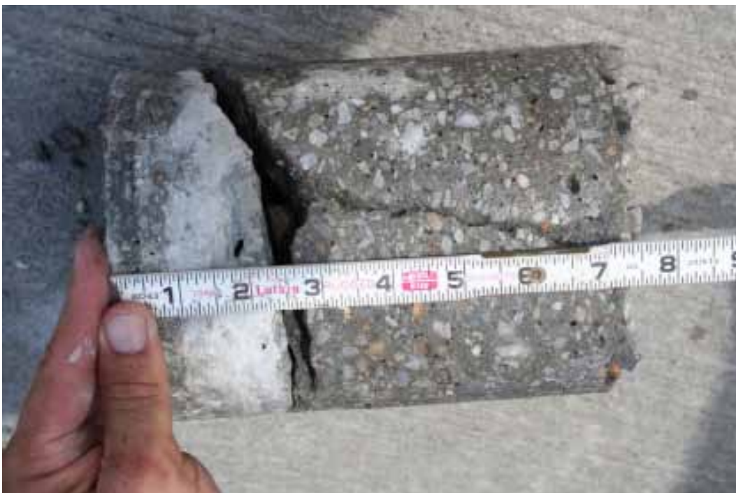
Figure 171. Core 1 from Crater 2 above pressure cell in traffic lane CeraTech Pavemend EX-H.
