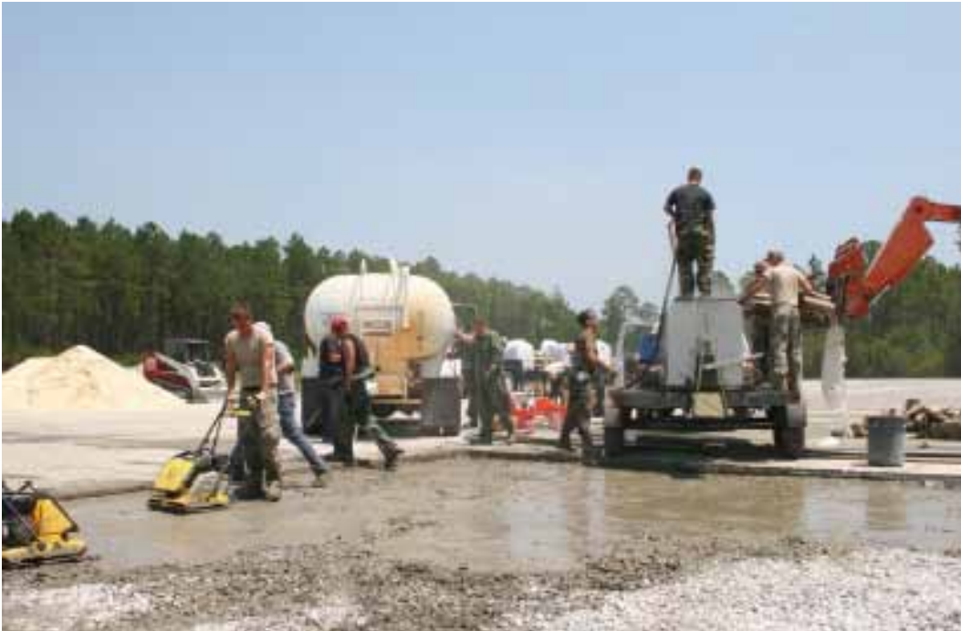
Figure 32. Vibratory plate compactors used to vibrate stone into grout mixture in Crater 1.
