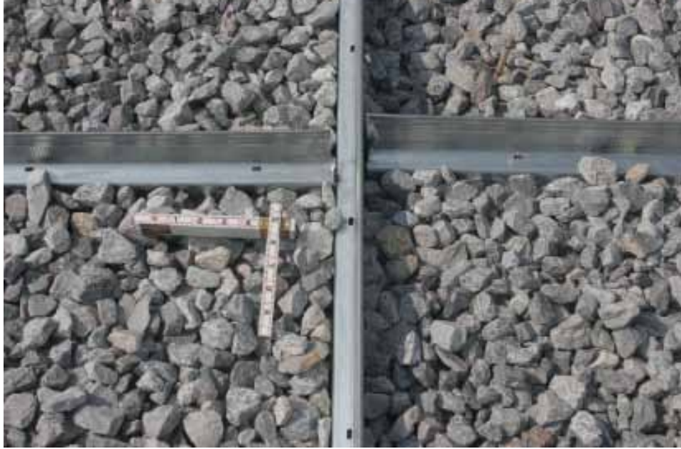
Figure 91. Photograph at the center of Crater 3 showing the stay-in-place forms and the #4 rock.
