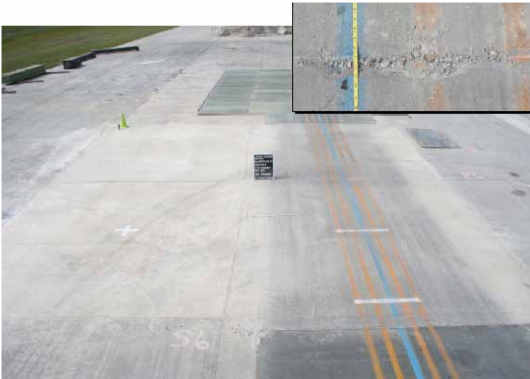
Figure 145. Crater 6 after 528 completed load cart passes.
