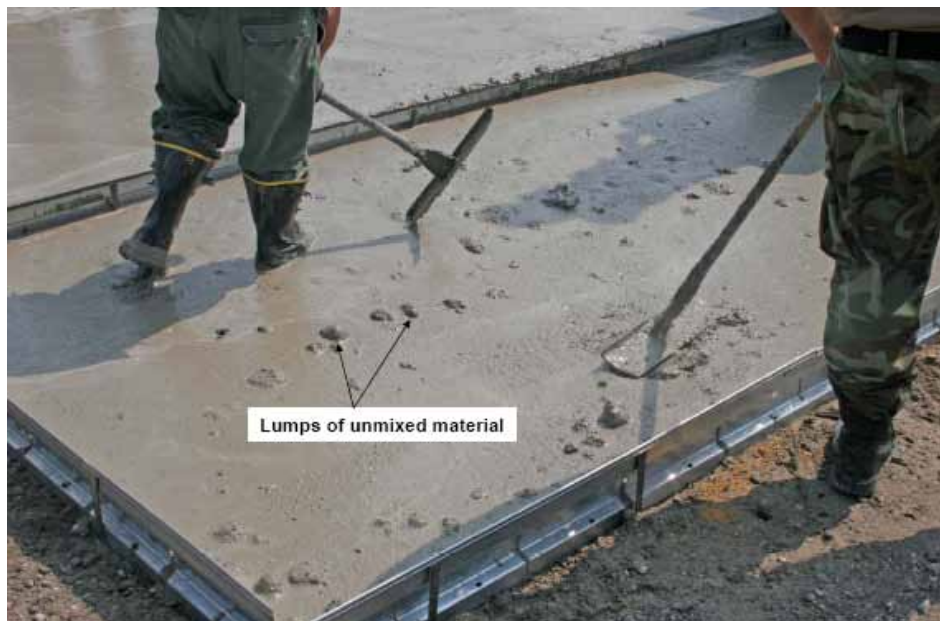
Figure 83. Batch 2 of Ultimax concrete, containing lumps of unmixed material, placed into Section 2 of Crater 4.
