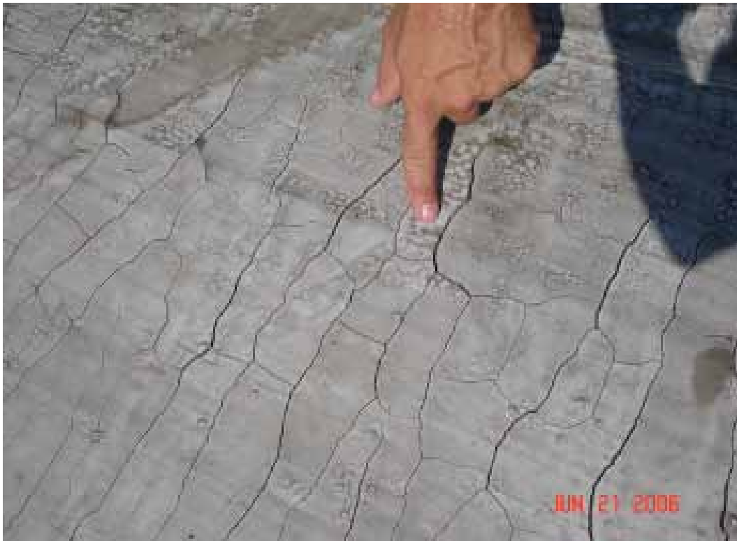
Figure 36. Shrinkage cracks in the surface of the stone and grout repair, Crater 1.
