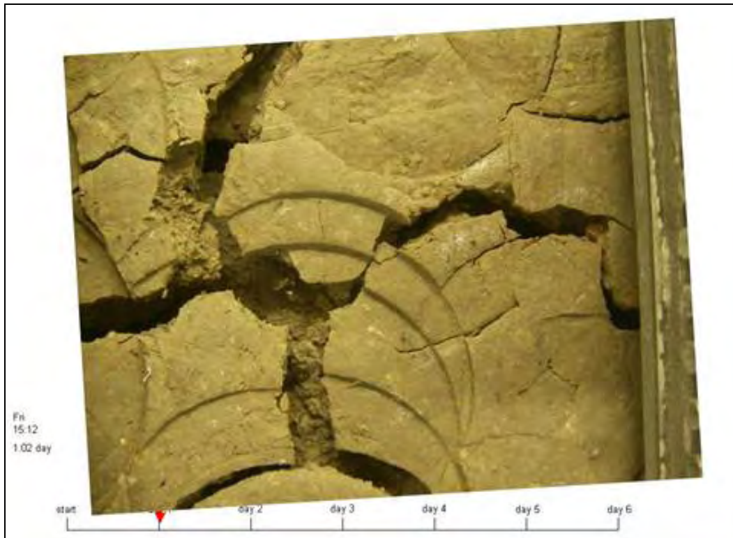
Figure 20. Image of cracks using digital camera.
