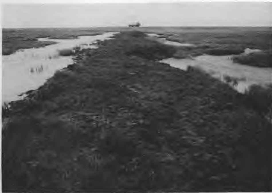
Figure 13. Surface of a peat road near the Putuligayuk River in the Prudhoe Bay oil field. The ponded water in the scraped areas creates wide barriers on both sides of the road. The water has also eroded the road bed, making it impassable. These surfaces are very slow to revegetate; this road is at least 15 years old. Most of the plant cover is mosses (e.g. Bryum spp. and Ceratodon purpureus). The vascular taxa include Carex aquatilis, Braya pilosa, Deschampsia caespitosa, Puccinellia andersonii, Draba alpina, Saxifraga hirculis and S. oppositifolia. (Photo by D.A. Walker, 31 July 1983.)
