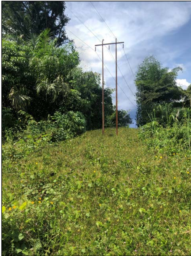
Figure 40: Visualisation of the 33 kV transmission line.
