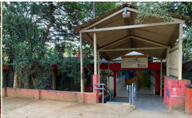
EMEF Campos Salles school front entrance. The image highlights the removal of the external walls.
