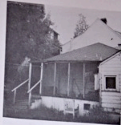
2631 CHANNING . . . . . THE STAIRS ARE COLLAPSING & ROT IS CREEPING UP THE PORCH. SMALL WONDER THE UNIVERSITY IS ENTERING THE STUDENT HOUSING FIELD.
