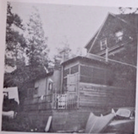
2635 CHANNING . . . . . THE REAR A CLAPTRAP OF SUB-STANDARD ADDITIONS. THE WHOLE A SERIOUS FIRETRAP. ANOTHER EXAMPLE OF STUDENT HOUSING IN BERKELEY.
