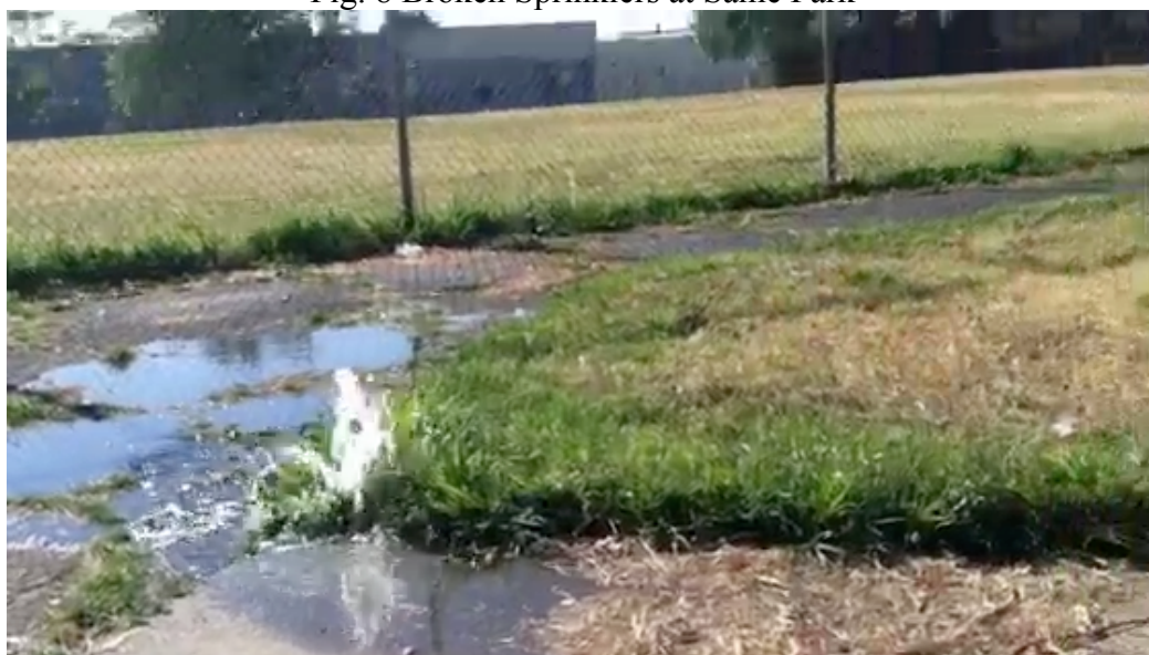
Fig. 8 Broken Sprinklers at Same Park
