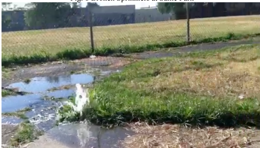
Fig. 8 Broken Sprinklers at Same Park
