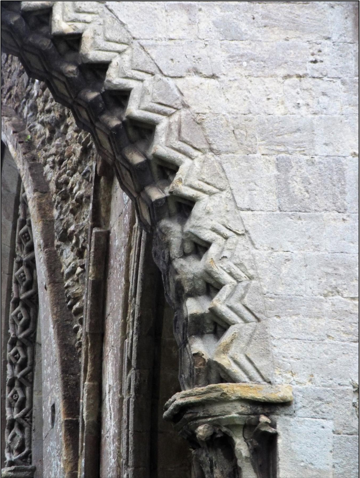
Figure 7.8: detail, northeast crossing pier of abbey church, looking east. (photo by Ross McIntire)
