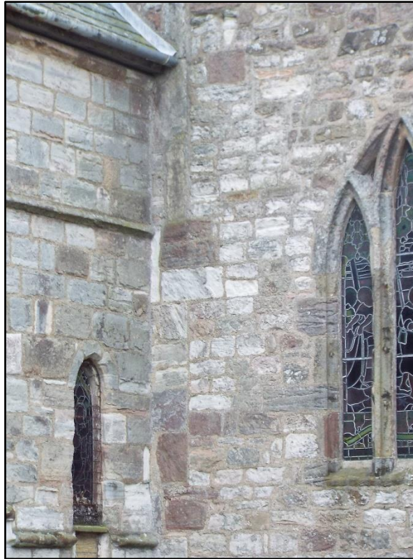
Figure 6.14: The join between the northeast corner of the original nave and the later north aisle and chancel of St Mary's Church, Lindisfarne. Parts of the irregularly arrangement of the quoin stones of the nave can still be seen, suggesting that the nave was built in the eleventh century. (Photo by Ross McIntire)
